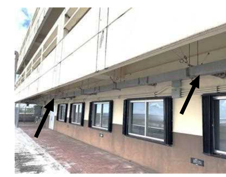
EXISTING EXTERIOR SUSPENDED AC DUCTING
