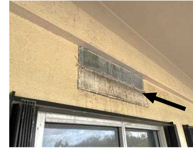
DETERIORATED EXHAUST/OUTSIDE AIR GRILLE COVER.
