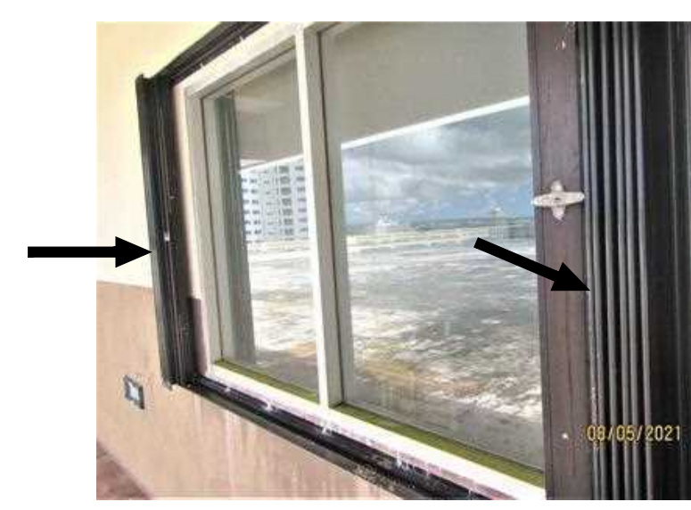
DETERIORATED WINDOW ACCORDION SHUTTER
