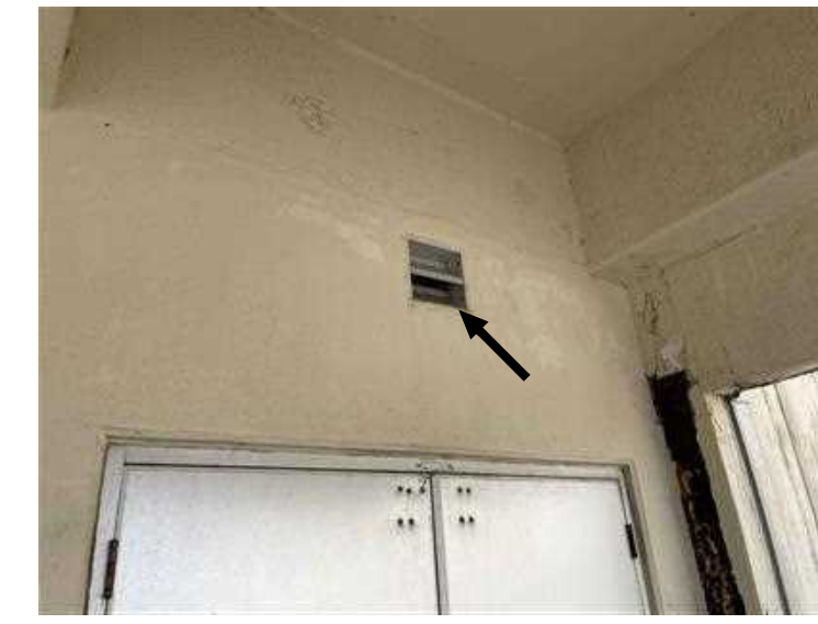
DETERIORATED WALL OUTSIDE AIR GRILLE.
