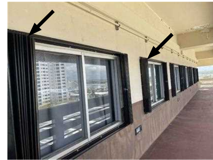
DETERIORATED WINDOW ACCORDION SHUTTERS (TYP 30 PLACES).
