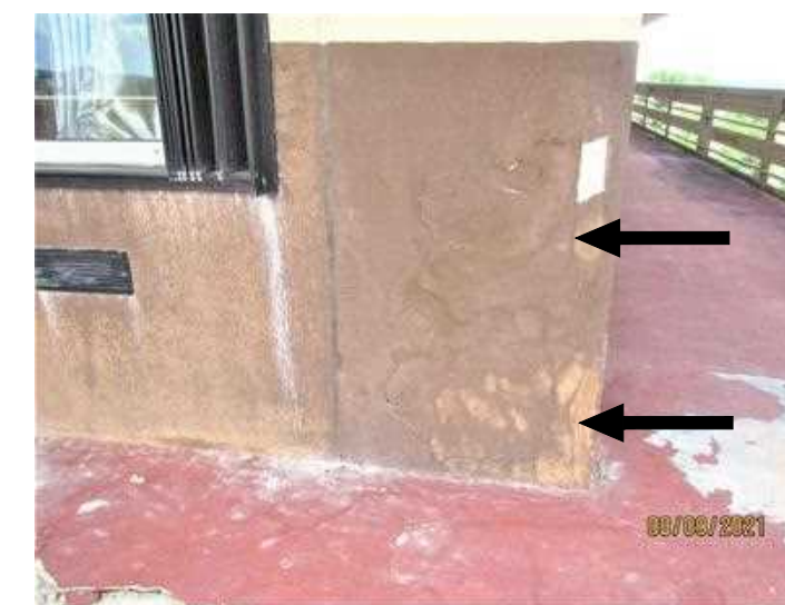
COLUMN SPALLS (10 SF)
