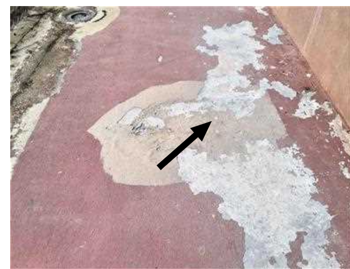
CONC SPALLS ON FLOORS (4 Sf)
