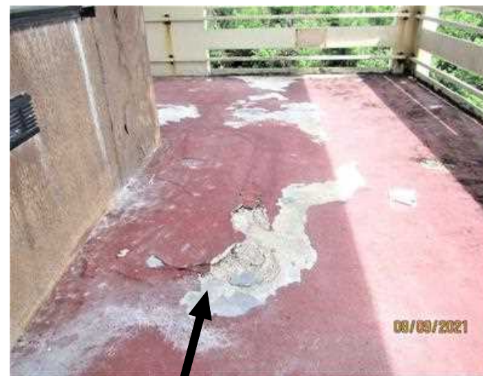
FLOOR BUCKLING SPALLS (42 Sf + 225 Sf + 75 Sf + 32 Sf) = 374 Sf
