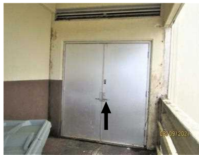
DETERIORATED DOOR SEALANT & SEAL (40 Lf, 45 Lf)
