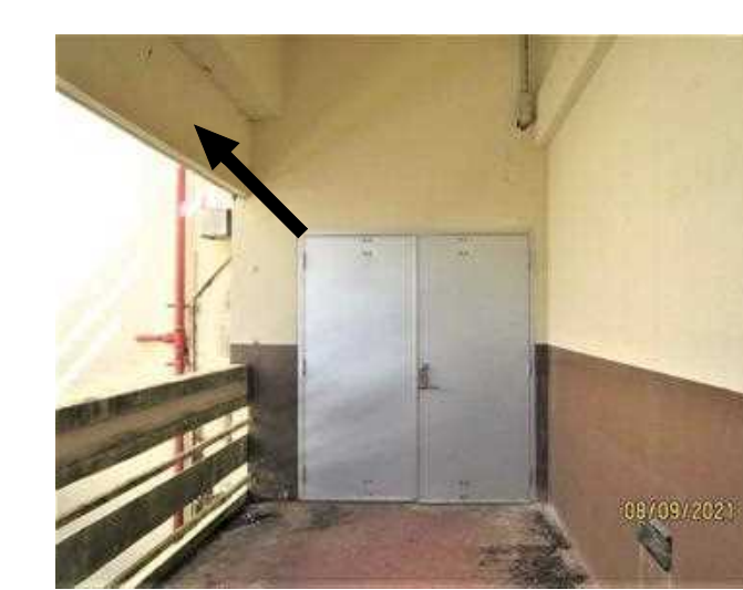
CONC SPALLS ON PARAPET (4 Lf)
