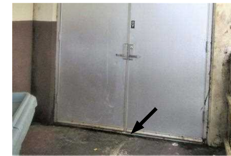
DETERIORATED DOOR THRESHOLD (6 Lf)
