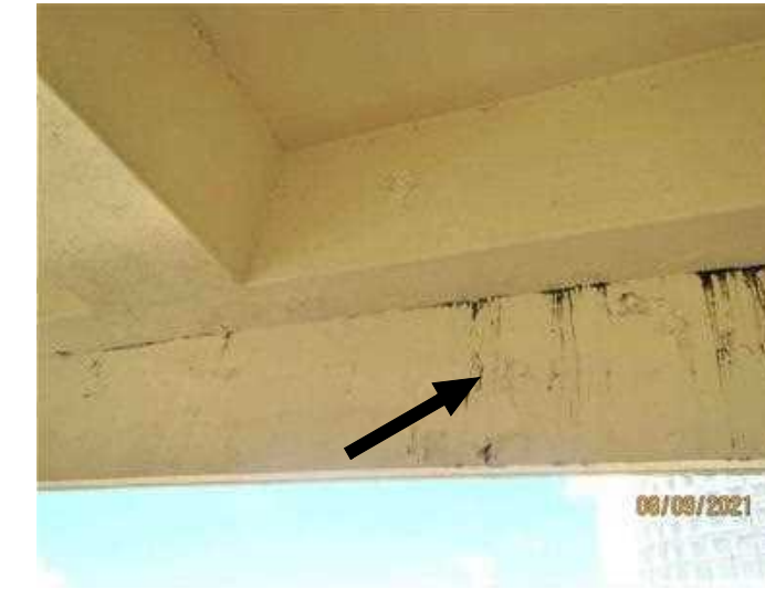
PAINT FLAKING AT SOFFIT FASCIA (60 Sf)
