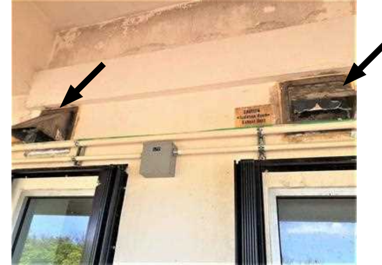
DETERIORATED EXHAUST HOOD (7 ea).
