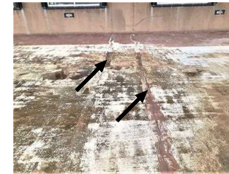
ROOF CRACKS ON SLAB (38 lf).
