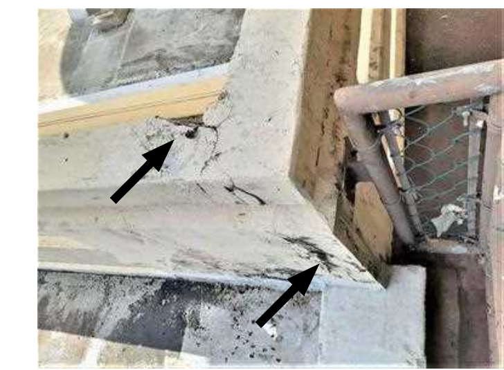
CONCRETE SPALLS ON PARAPET (8 sf).
