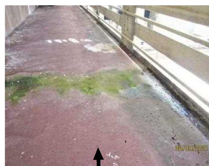
DETERIORATED CORRIDOR FLOOR COATING MEMBRANE (2,480 SF)
