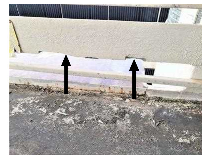
CONC RAILING SPALLS (8 Lf x 6")
