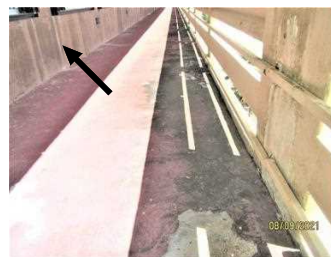
DETERIORATED WALL PAINT (3,510 Sf)
