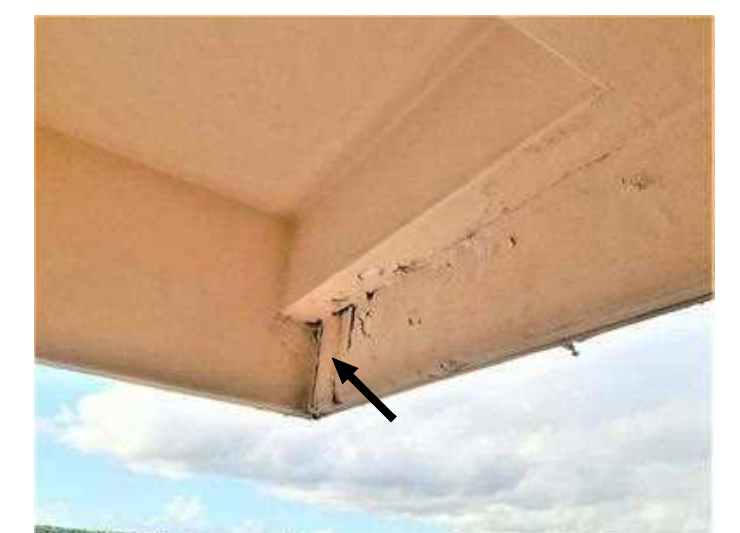
CRACK AT SOFFIT CORNER (2 Lf)
