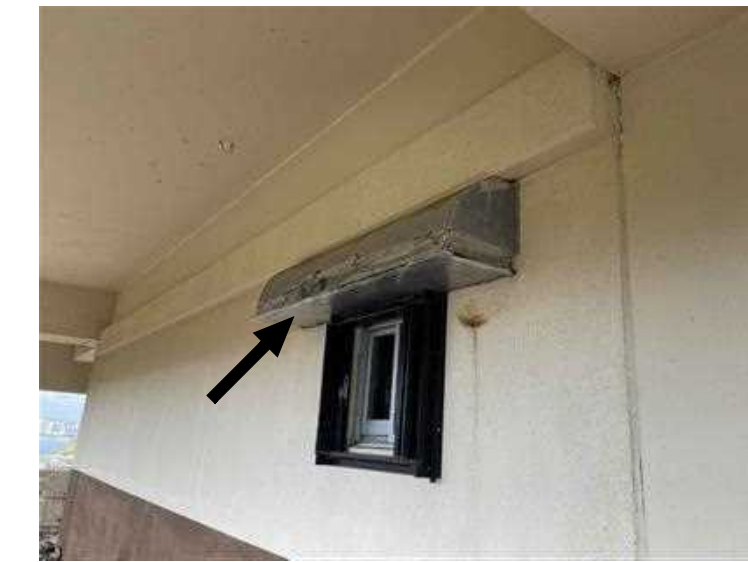
DETERIORATED WALL EXHAUST HOOD.
