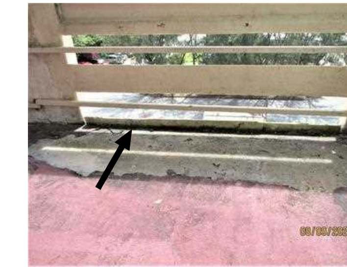
CRACKS ON PARAPET RAILINGS (2 Lf)
