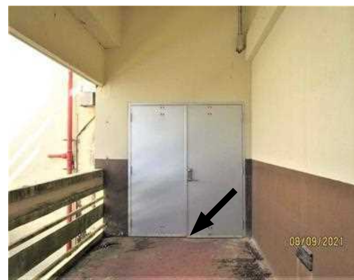
DETERIORATED DOOR THRESHOLD (12 Lf)
