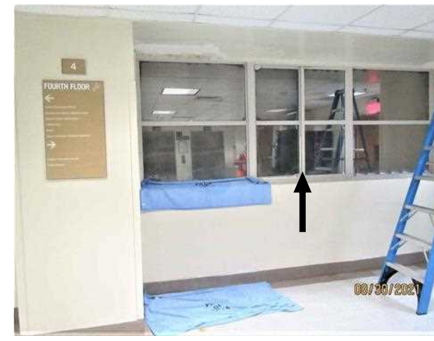
DETERIORATED GLASS WINDOW AND FRAMES
