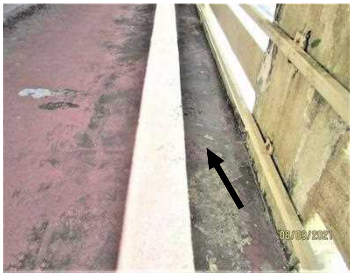
FLOOR DIRT WITH ALGAE (114 Sf)
