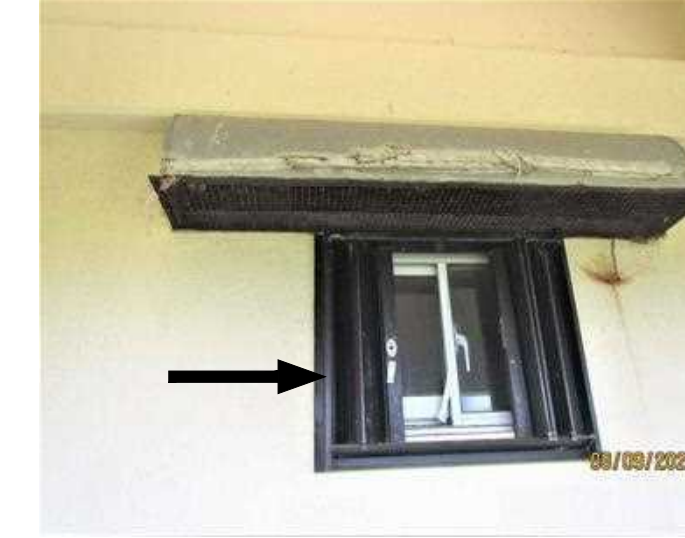
DETERIORATED WINDOW SHUTTERS (TYP 23 PLACES)
