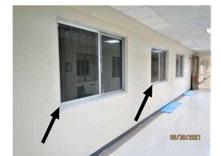
DETERIORATED WINDOW FRAME, GLASS, SEAL & SEALANT
