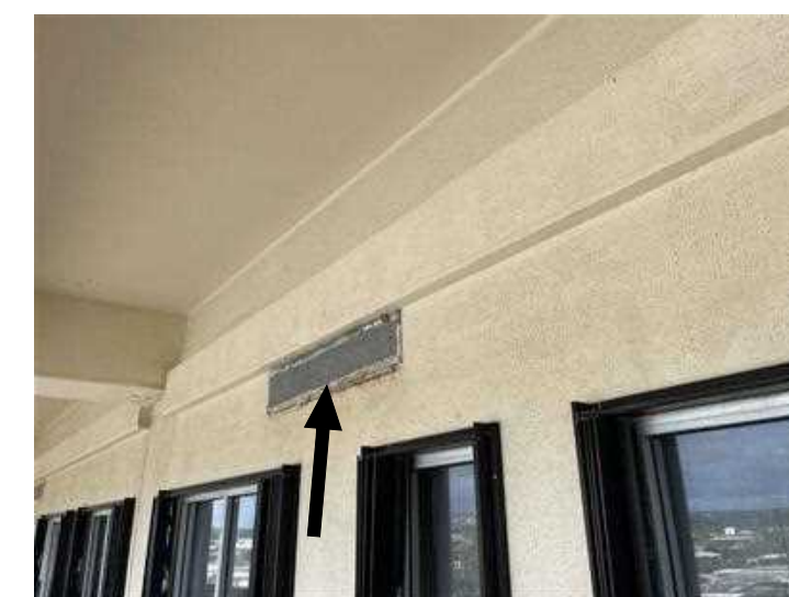
DETERIORATED EXHAUST/OUTSIDE AIR GRILLE COVER.
