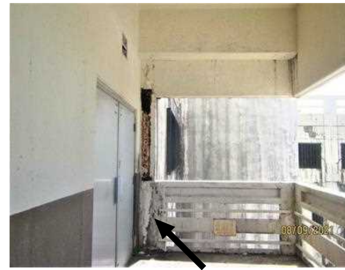
COLUMN SPALLS (2 sf).
