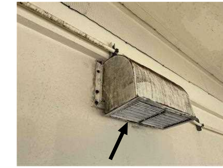
DETERIORATED WALL EXHAUST HOOD.
