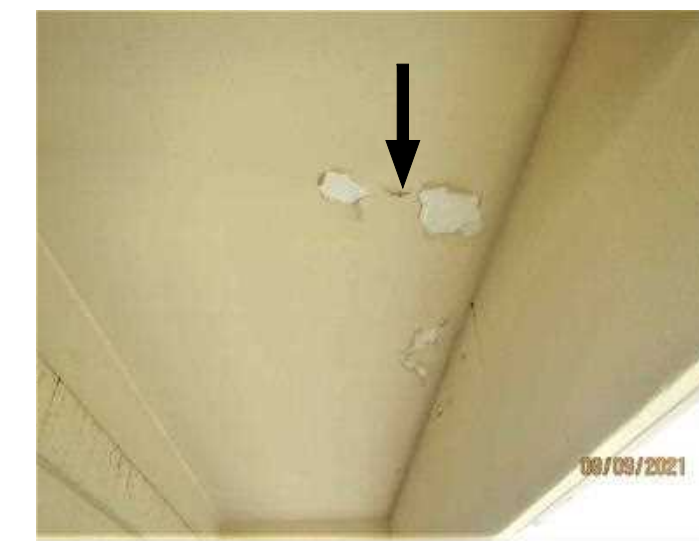
PAINT FLAKING AT SOFFIT CEILING (240 Sf + 240) = 480 Sf
