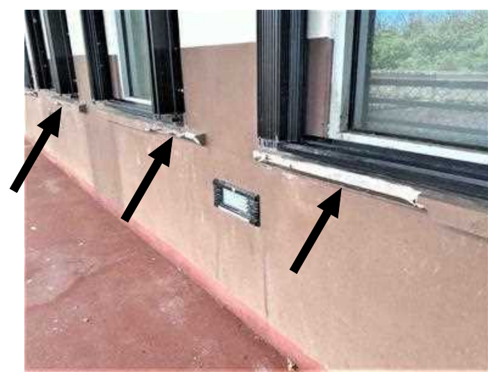
CONCRETE SPALLS ON WINDOW SILL TRIM (12 sf).
