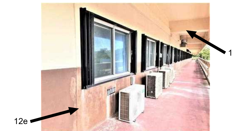
12e DETERIORATED WALL PAINTS (1,040 sf). 13e DETERIORATED CEILING PAINTS (640 sf).
