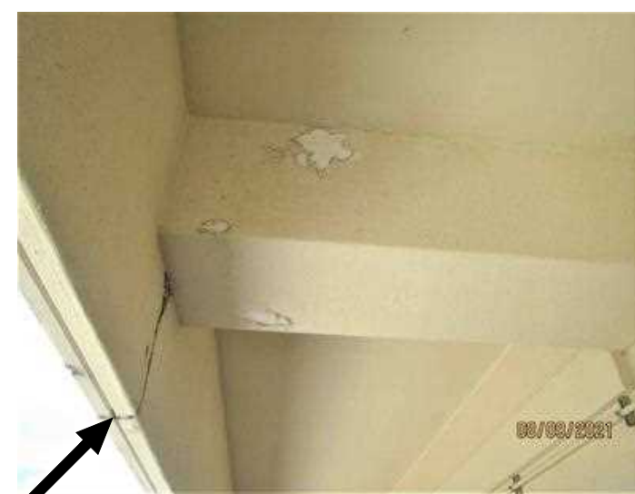
CRACKS AT PARAPET WALL JOINT (6 LOC)
