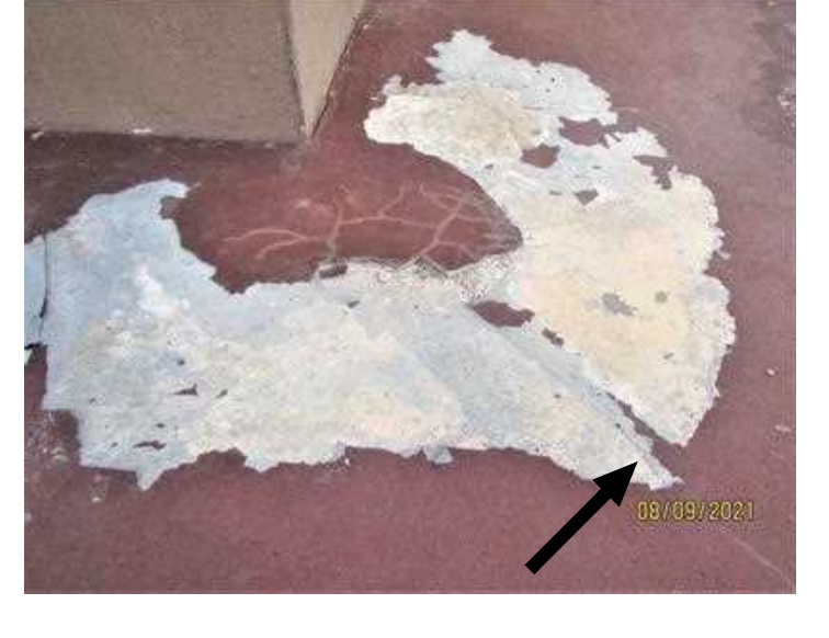
FLOOR CRACKS (16lf).
