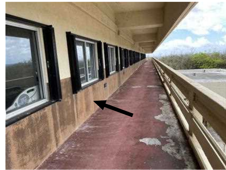
DETERIORATED WALL, and PARAPET WALL PAINTS.
