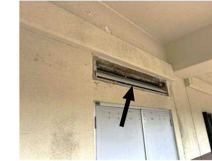
DETERIORATED EXHAUST/OUTSIDE AIR GRILL
