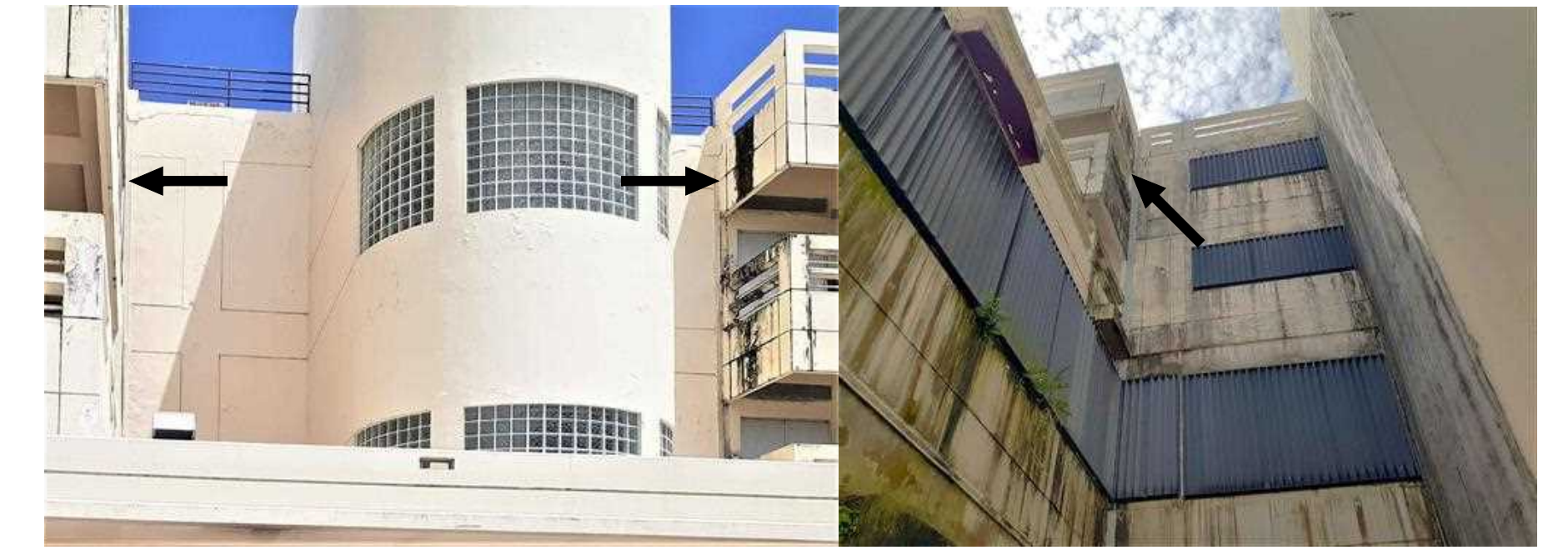
DETERIORATED VERTICAL SEISMIC JOINT, TYPICAL 4 PLACES (52 Lf)
