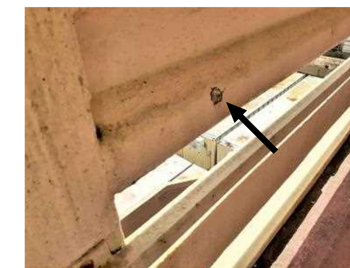
CONC FLAKING ON RAILING (2 Sf)
