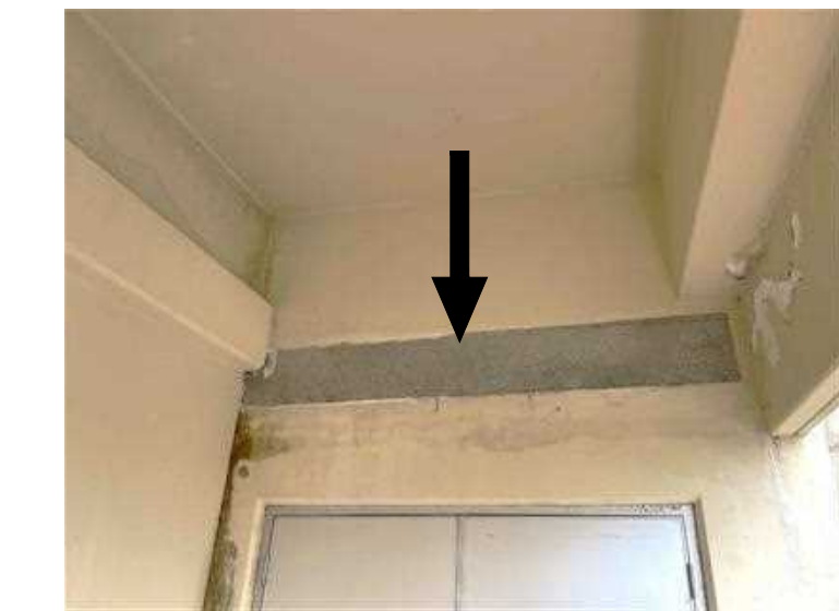
EXISTING WALL, EXHAUST HOOD MISSING.
