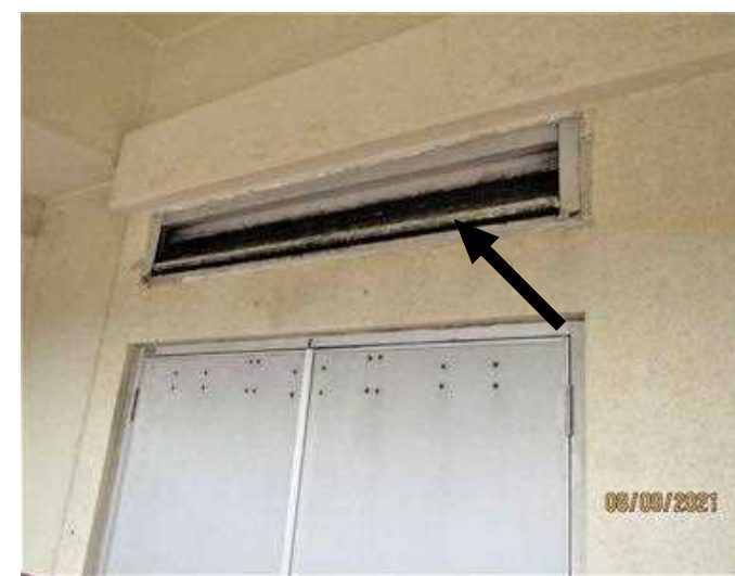
BROKEN OVERHEAD DOOR AIR INTAKE
