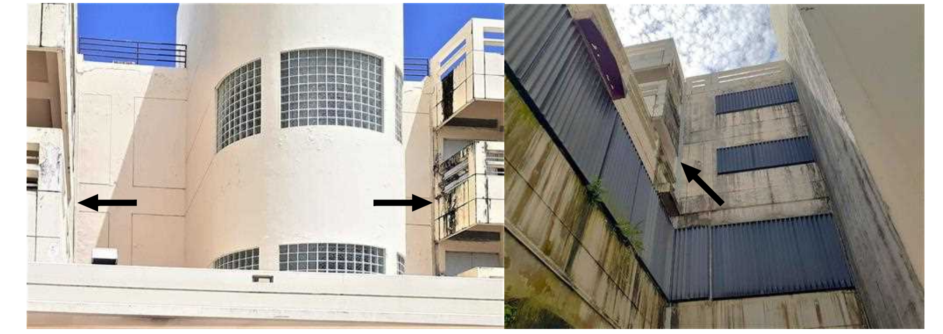
DETERIORATED VERTICAL SEISMIC JOINT, TYPICAL 4 PLACES (52 Lf)
