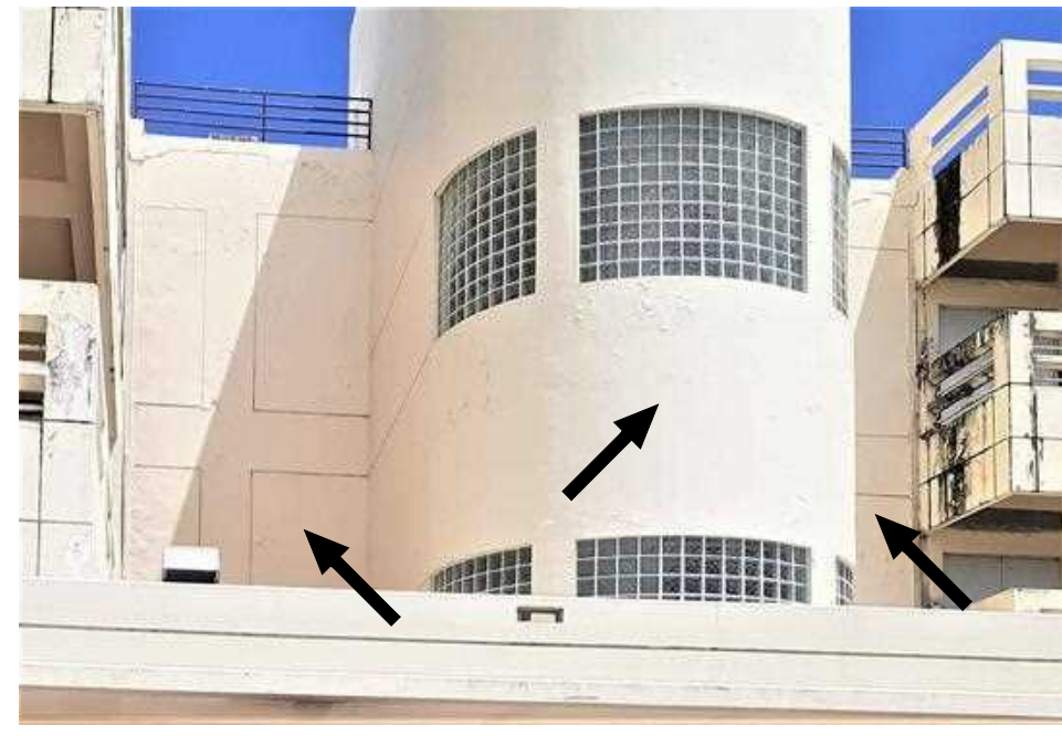
DETERIORATED EXISTING WALL PAINTS (1118 sf).
