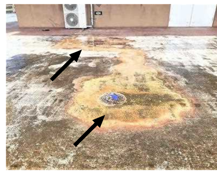
ROOF DRAIN WATER PONDING (4 ea) 860 sf.
