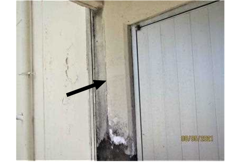
CRACKS ON WALLS (13 lf).
