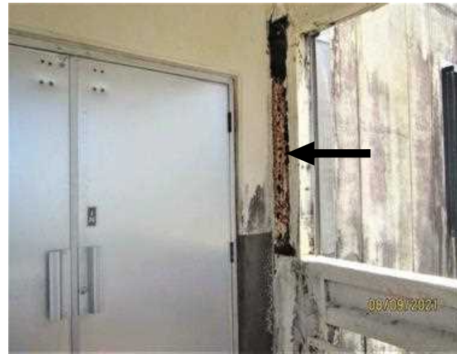
DETERIORATED STEEL PILASTER (10 lf).
