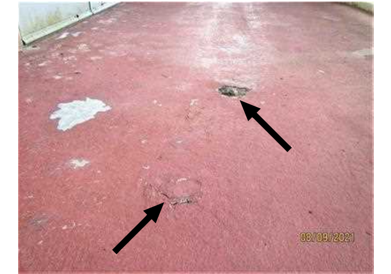
CONC SPALLS ON FLOOR (16 Sf)
