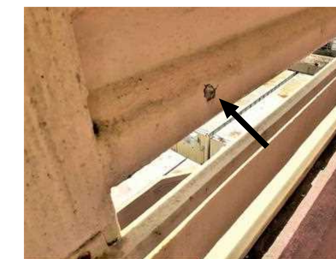
CONC FLAKING ON RAILING (2 Sf)
