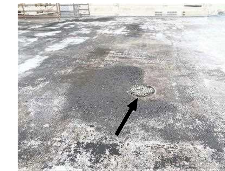
DETERIORATED ROOF DRAIN STRAINER (4 ea).
