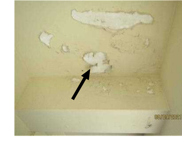
PAINT FLAKING ON CEILING (70sf).
