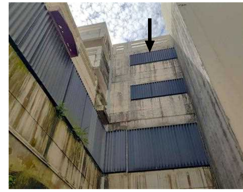
DETERIORATED ACCORDION WINDOW SHUTTER
