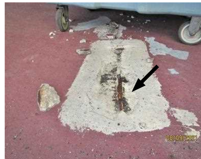
FLOOR SPALL WITH EXPOSED REBAR (20sf).
