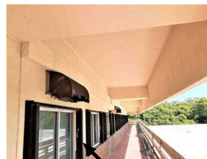
DETERIORATED WINDOW SHUTTERS (TYP 14 PLACES)
