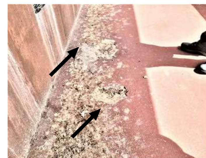
BIRDS DROPPINGS AT CORRIDOR (240 Sf) BIRD DROPPINGS FROM BEAM LEDGES ABOVE, ETC
