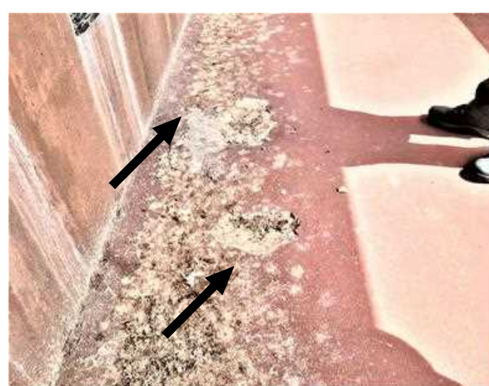
BIRDS DROPPINGS AT CORRIDOR (240 Sf) BIRD DROPPINGS FROM BEAM LEDGES ABOVE, ETC
