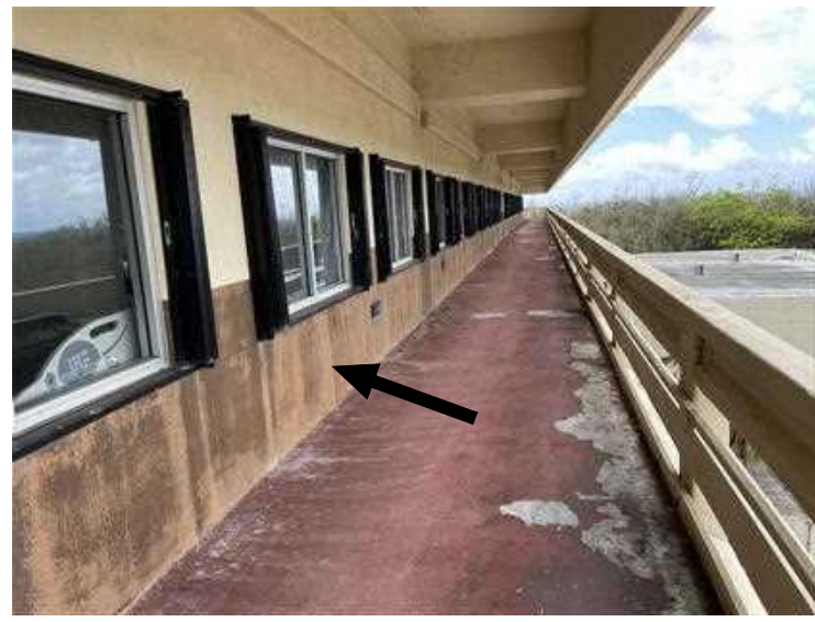
DETERIORATED WALL, and PARAPET WALL PAINTS.
