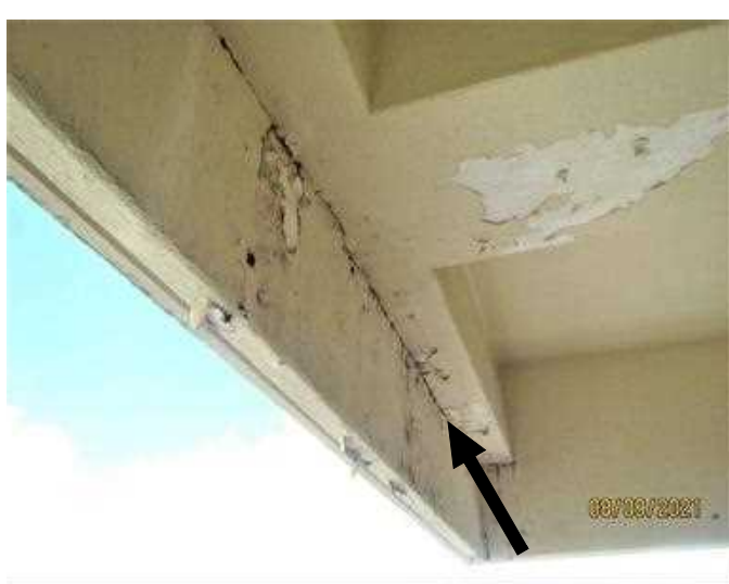
PAINT FLAKING AT SOFFIT (16 Sf)
