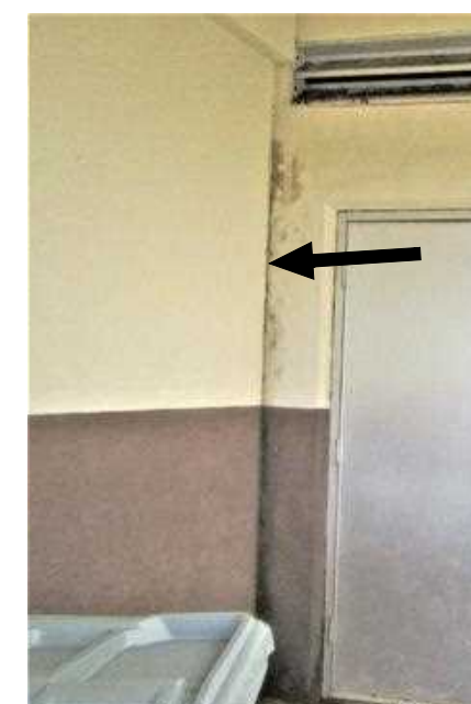
WALL CRACKS (9 Lf)
