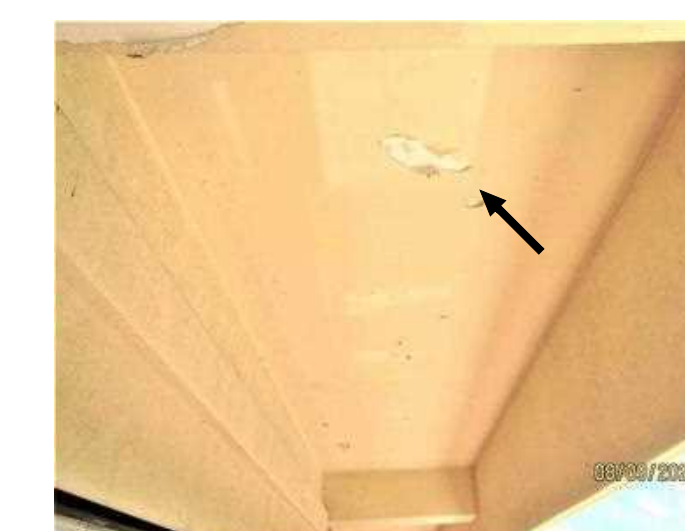
PAINT FLAKING AT CEILING (31 Sf)
