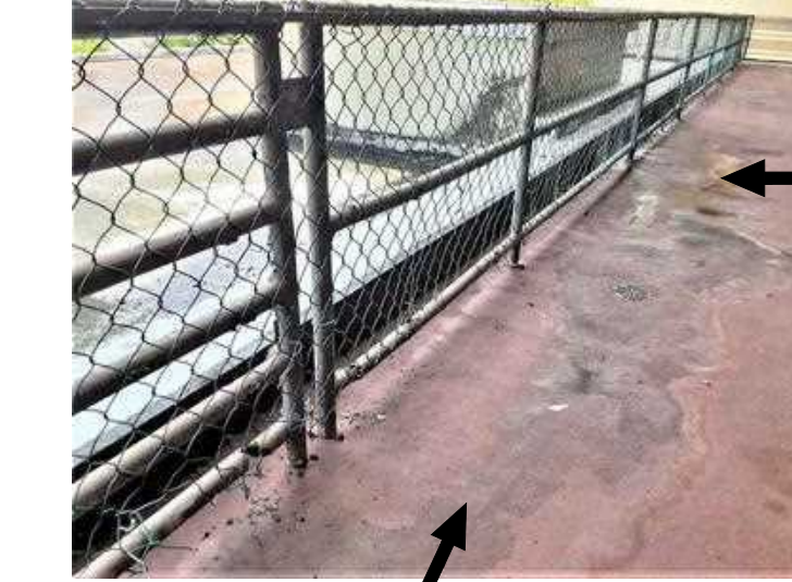
WATER PONDING WITH GREEN ALGAE (392 sf).
