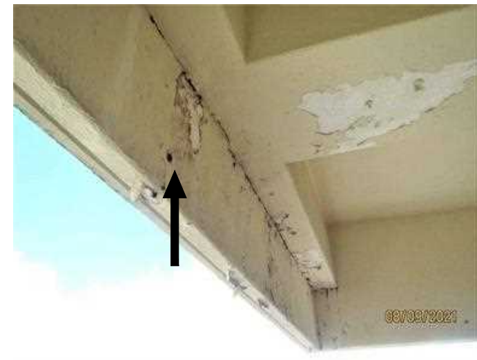
SPALL WITH EXPOSED REBAR AT SOFFIT FASCIA (2 Sf)
