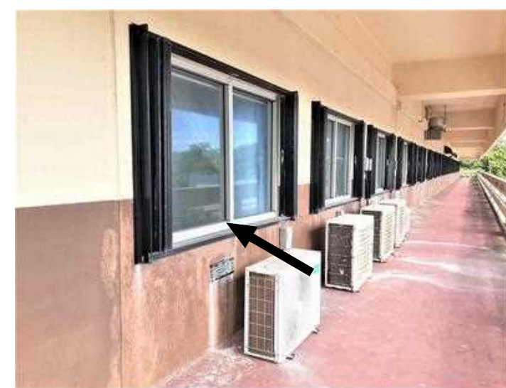
CONDENSATION AT WINDOWS (10 EA 6'x4') DETERIORATED SEAL (2 EA 28"x48")
