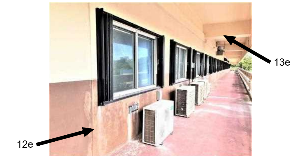
12e DETERIORATED WALL PAINTS (1,040 sf). 13e DETERIORATED CEILING PAINTS (640 sf).
