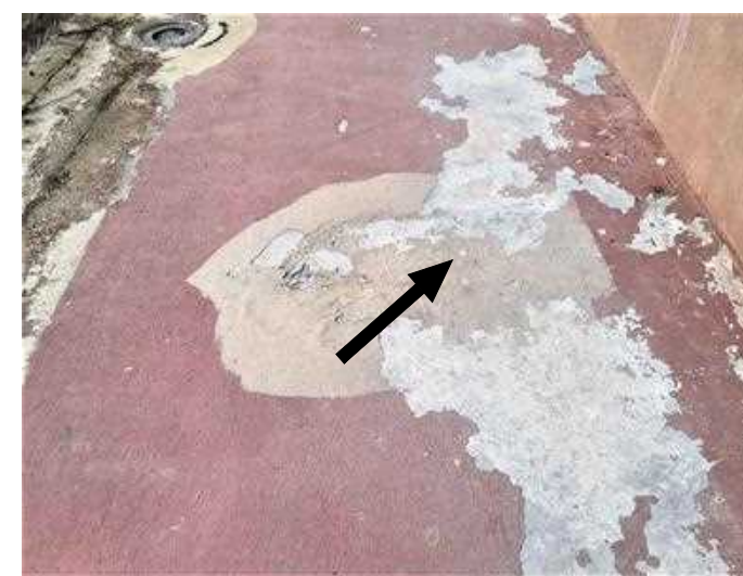
CONC SPALLS ON FLOORS (4 Sf)
