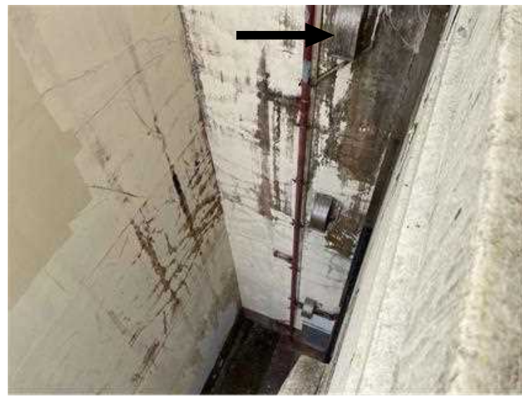
DETERIORATED WALL EXHAUST HOOD.
