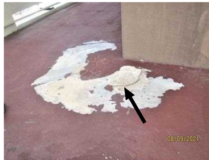
CONCRETE FLOOR SPALLS (12sf).
