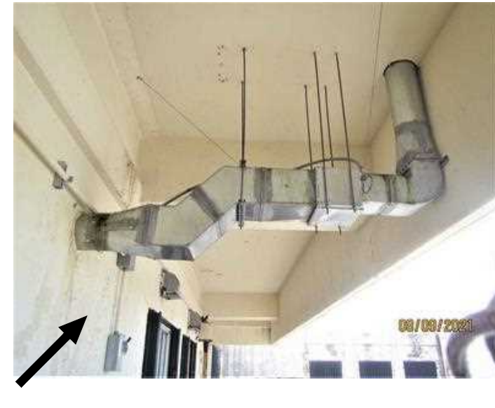
PAINT FLAKING ON WALL (50sf).
