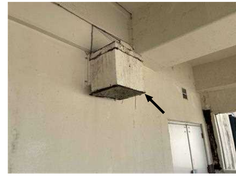
DETERIORATED WALL EXHAUST HOOD.
