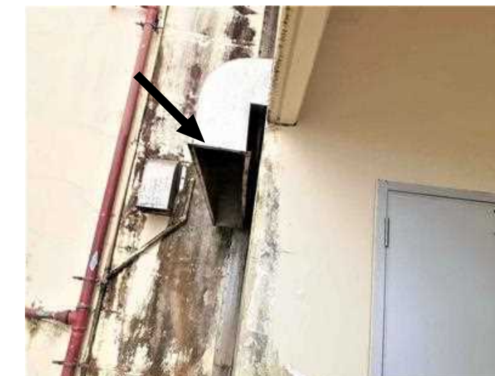
EXHAUST HOOD COVER MISSING
