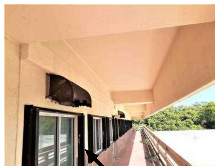
DETERIORATED WINDOW SHUTTERS (TYP 14 PLACES)
