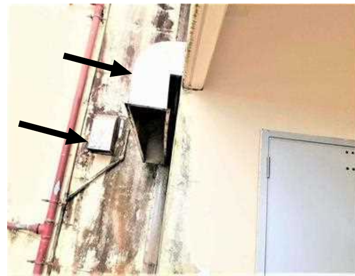
DETERIORATED EXHAUST HOOD
