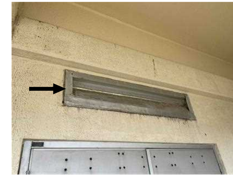
DETERIORATED WALL OUTSIDE AIR GRILLE.
