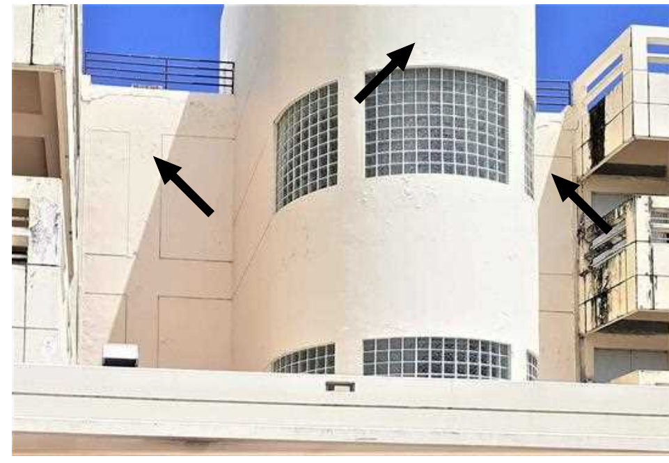
DETERIORATED EXISTING WALL PAINTS (1118 sf).
