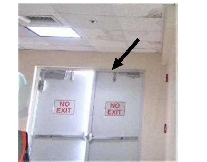
DETERIORATED DOOR SEAL & SEALANT (SEALANT 80 Lf) (SEAL 56 Lf)
