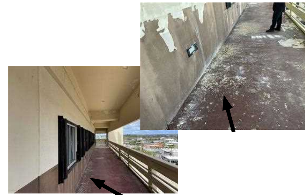
BIRDS DROPPINGS PRESENT ON BEAM, HOODS, PIPES, DUCT WORK, SHUTTER HEAD, ETC. FROM LIGHT TO HEAVILY INFESTED NARROW TO EXTRA WIDE AREAS.
