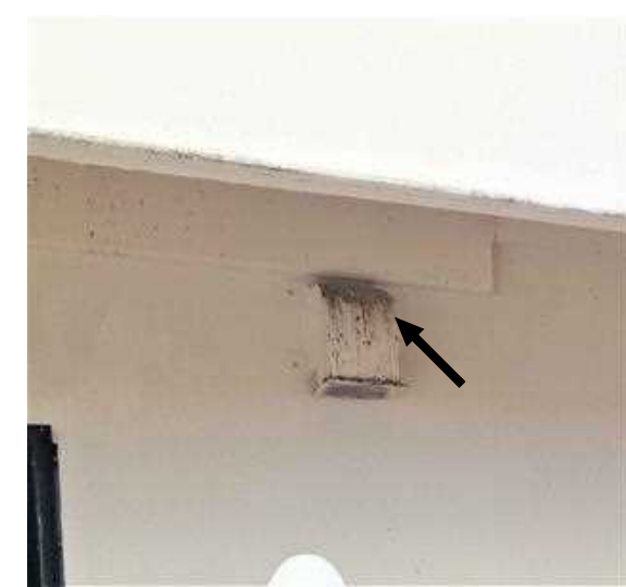
BIRD DROPPINGS PRESENT ON HOOD.
