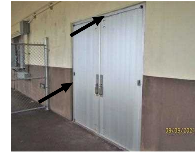
DETERIORATED DOOR SEALANT & SEAL (160lf SLNT, 112lf SEAL).
