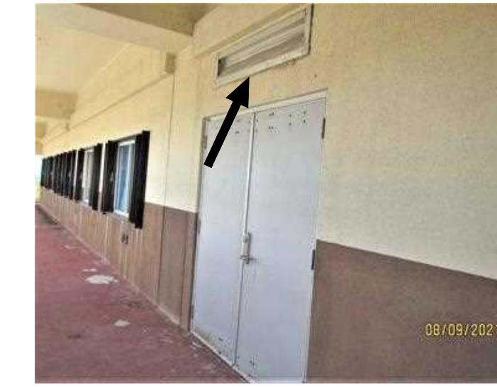
DETERIORATED OVERHEAD DOOR AIR INTAKE & GRILLE
