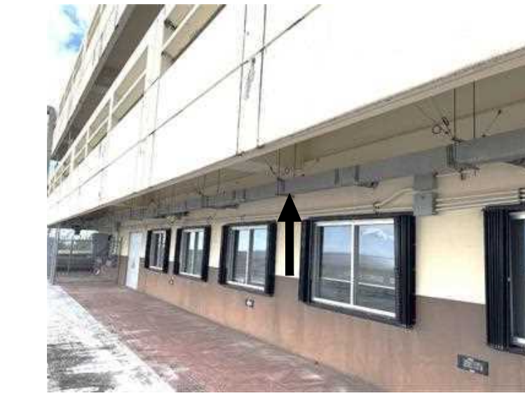
EXISTING DUCT WORKS.
