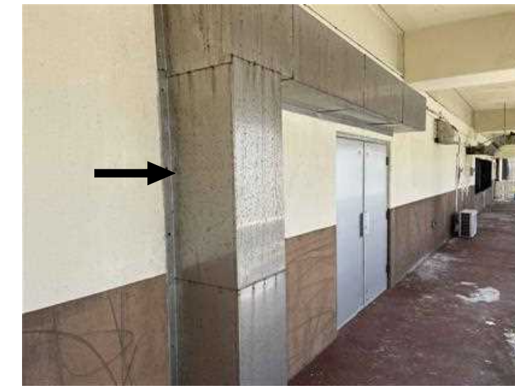
DETERIORATED WALL EXHAUST DUCT WORK.
