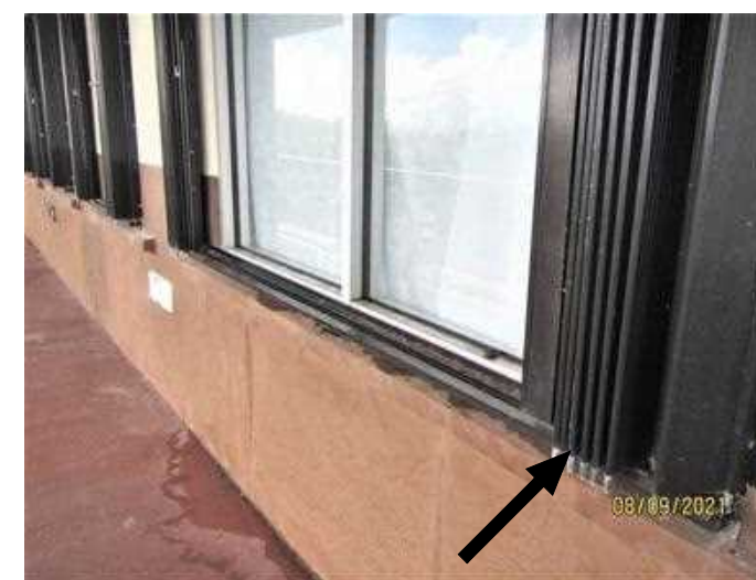
DETERIORATED WALL PAINT (3,510 Sf)
