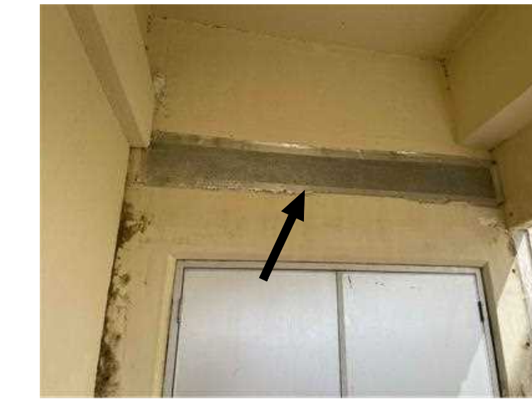
DETERIORATED EXHAUST/OUTSIDE AIR GRILLE COVER.
