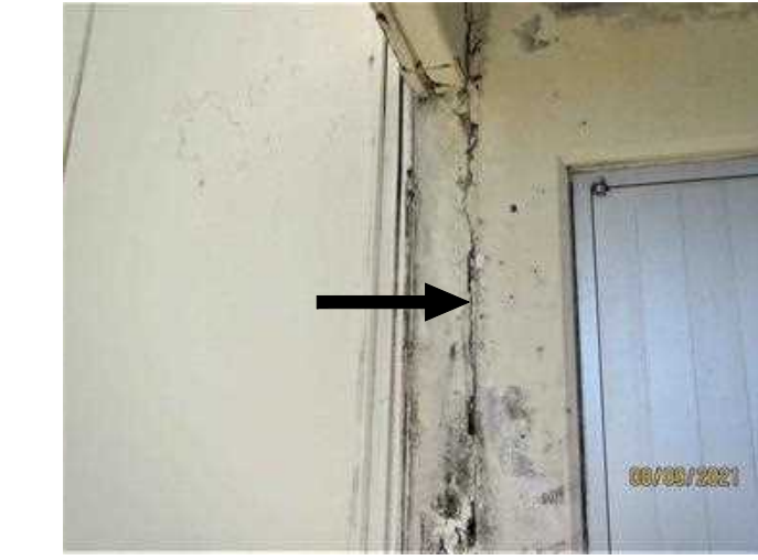
WALL CRACKS (16lf).
