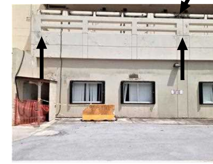
DETERIORATED PARAPET WALL PAINTS (1440 sf).
