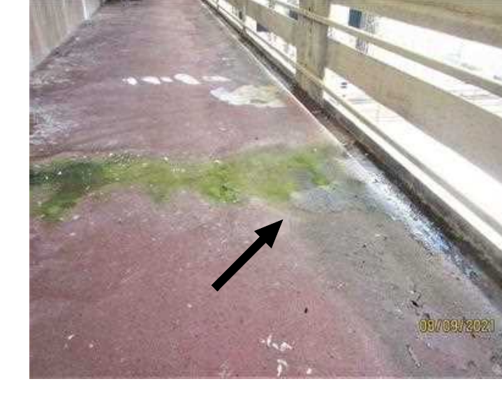
FLOOR DIRT WITH GREEN ALGAE (50sf).
