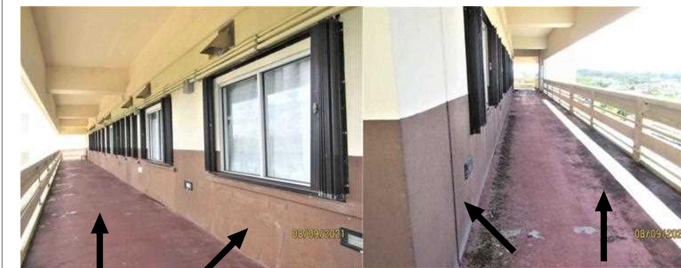
DETERIORATED WALL PAINT (3,510 Sf) DETERIORATED CORRIDOR FLOOR COATING MEMBRANE (1,496 Sf)
