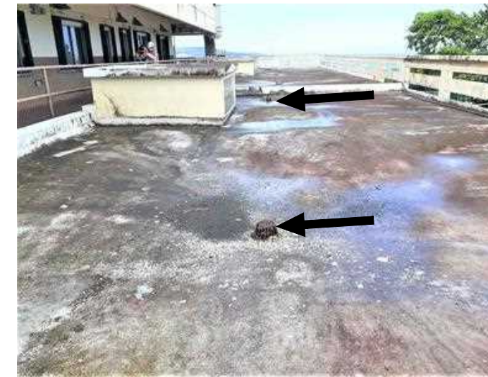
DETERIORATED ROOF DRAIN DOME COVER (6 ea).
