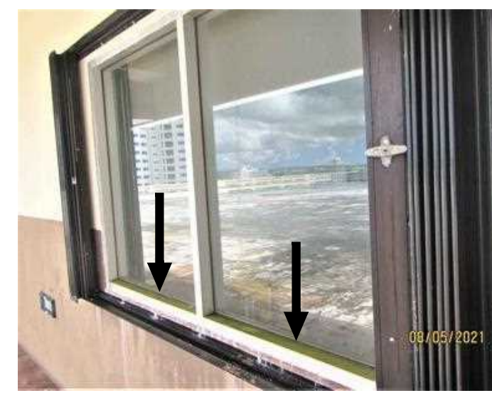
DETERIORATED WINDOW SEALANT & SEAL (248+240+160+128 SLNT) (48+32+48+32 SEAL).
