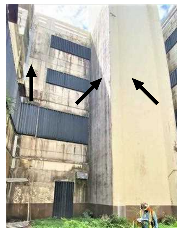
DETERIORATED EXISTING WALL PAINTS (900 sf).
