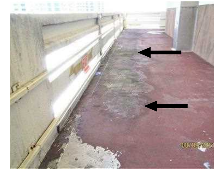
FLOOR PONDING (810sf)
