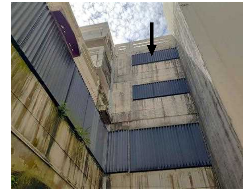
DETERIORATED ACCORDION WINDOW SHUTTER
