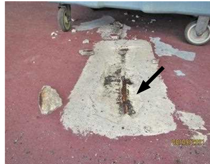
CONC SPALLS ON FLOOR WITH EXPOSED REBAR (36 Sf)
