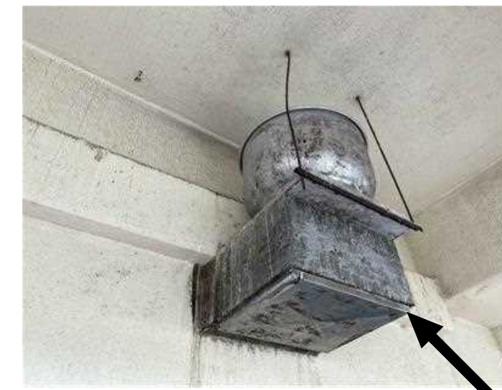
DETERIORATED WALL EXHAUST HOOD.
