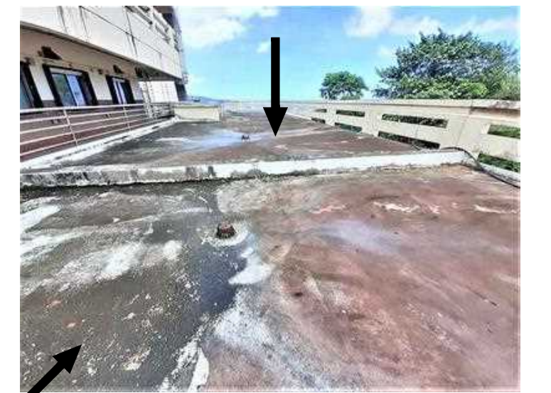
DETERIORATED ROOF COATING MEMBRANE (9900 sf).
