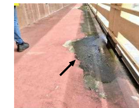
PONDING ON CORRIDOR (188 Sf)
