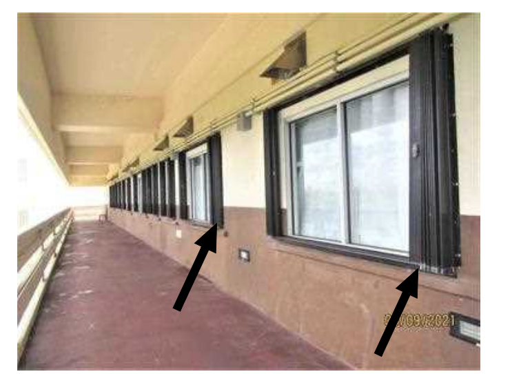
DETERIORATED WINDOW SHUTTERS (TYP 16 PLACES).
