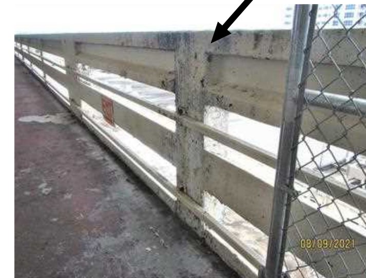
DETERIORATED PAINT & FLAKING ON CONCRETE RAILING/ PARAPET (1080sf).
