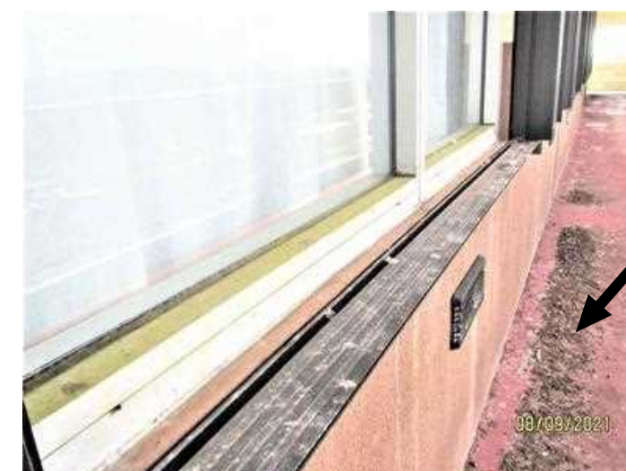
BIRD DROPPINGS FROM SHUTTER HEAD AND BEAM LEDGES, ETC.
