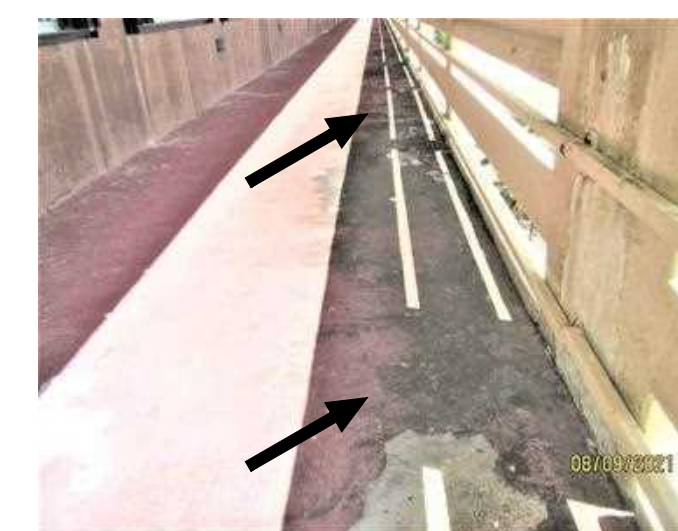
FLOOR WATER PONDING (450 Sf, 270 Sf, 114 Sf)
