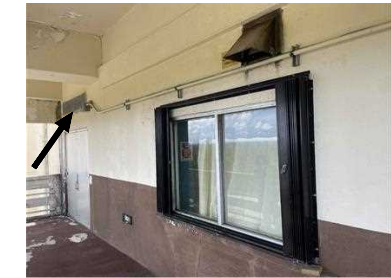
DETERIORATED EXHAUST/OUTSIDE AIR GRILLE COVER.
