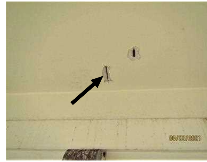
SPALLS ON CEILING (14sf).
