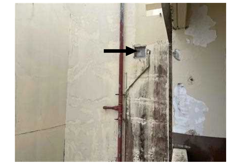
EXISTING WALL, EXHAUST HOOD MISSING.
