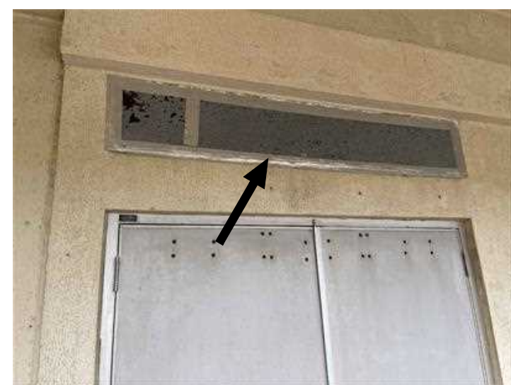
DETERIORATED EXHAUST/OUTSIDE AIR GRILLE COVER.
