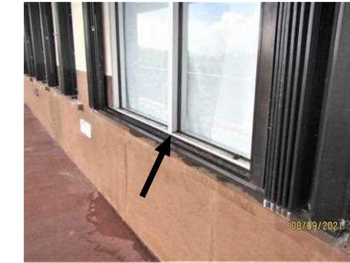
DETERIORATED WINDOW SEALANT & SEAL (573lf SEALANT, 573lf SEAL).
