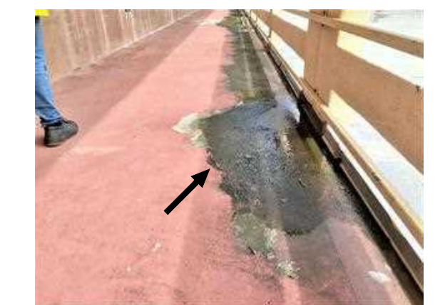
PONDING ON CORRIDOR (188 Sf)
