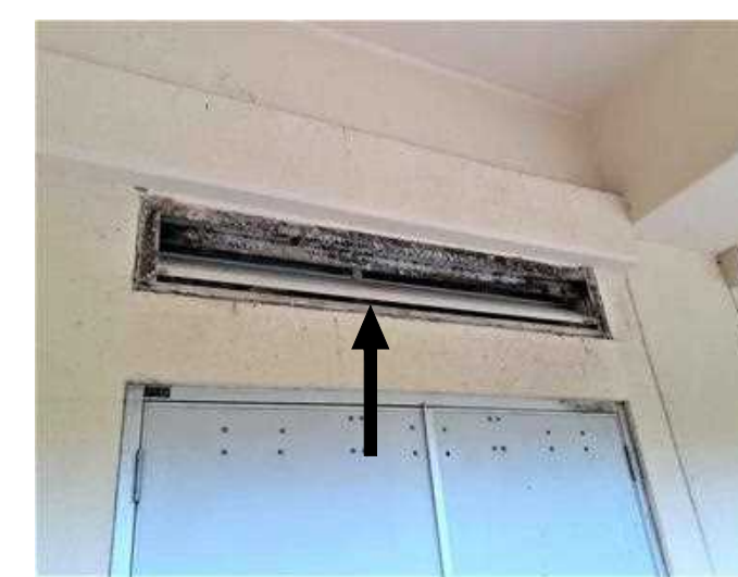
DETERIORATED DOOR HDR EXHAUST.
