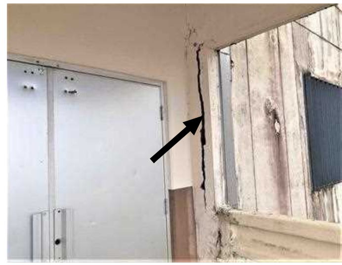
SEVERE CRACKS ON PILASTER WALL (13 lf).
