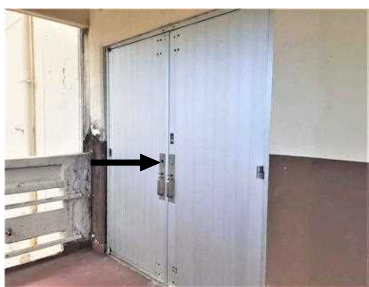
FAILED DOOR & ITS ACCESSORIES (1 ea).
