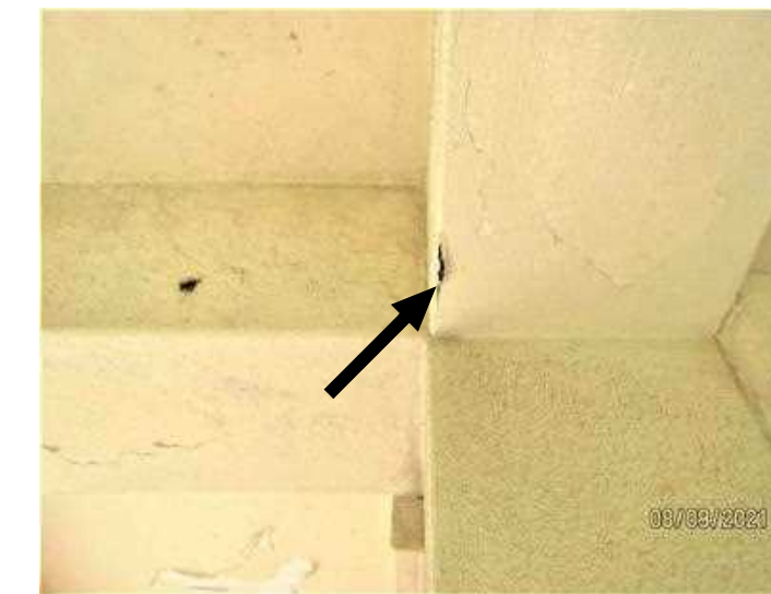
BEAM SPALLS (10 Sf)
