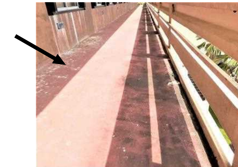
DETERIORATED FLOOR COATING MEMBRANE (640 sf).
