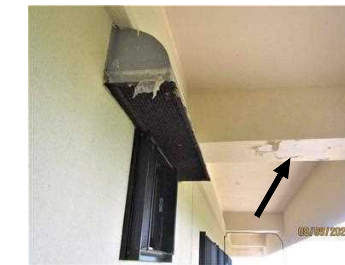
PAINT FLAKING AT BEAM (20 Sf)
