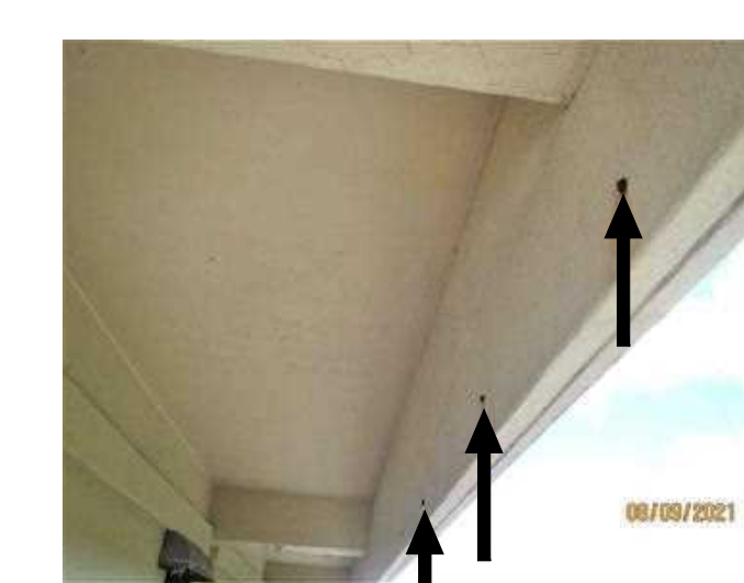
CORRODED BOLTS AT SOFFIT FASCIA (36 EA)
