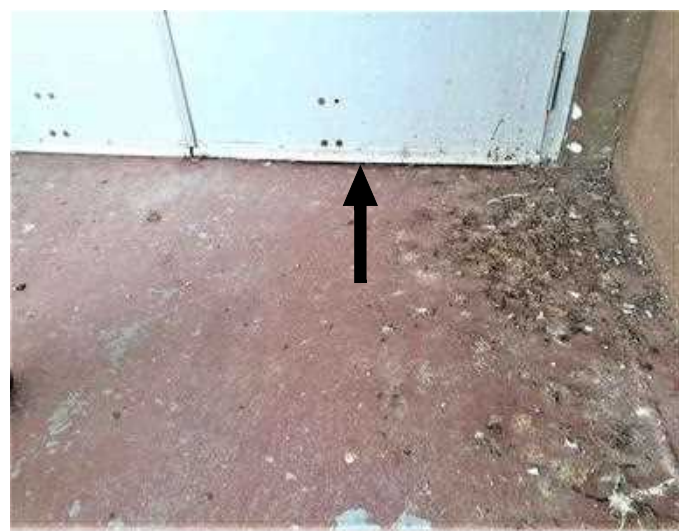
DETERIORATED DOOR THRESHOLD (12 Lf)
