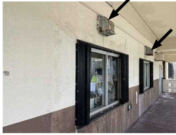
DETERIORATED WALL EXHAUST HOOD.
