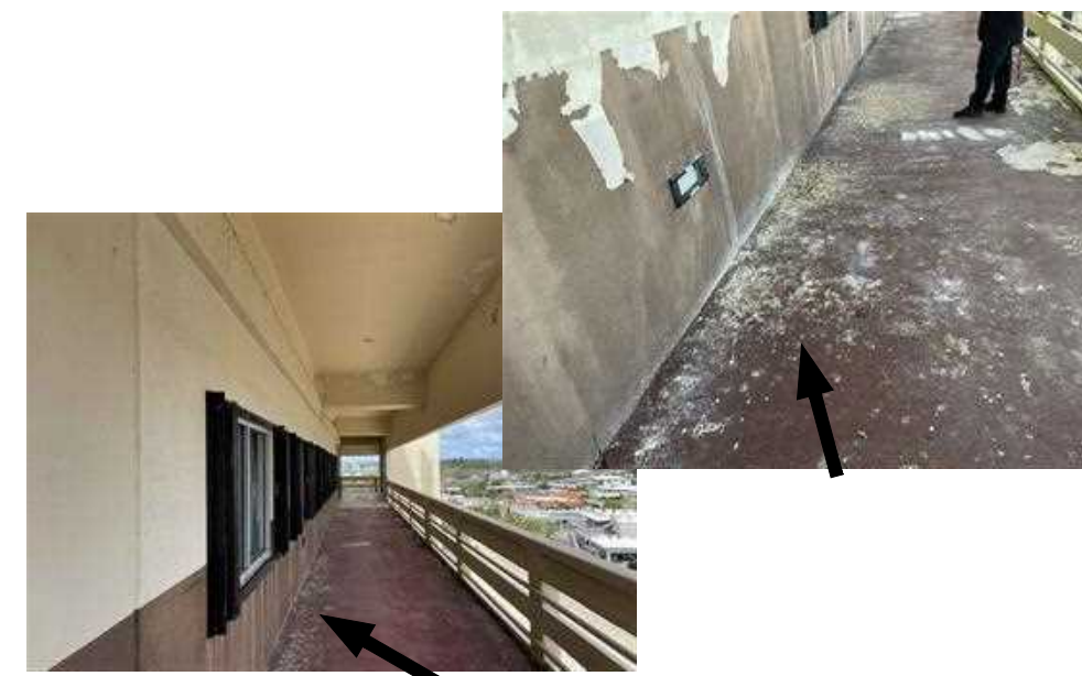
BIRDS DROPPINGS PRESENT ON BEAM, HOODS, PIPES, DUCT WORK, SHUTTER HEAD, ETC. FROM LIGHT TO HEAVILY INFESTED NARROW TO EXTRA WIDE AREAS.
