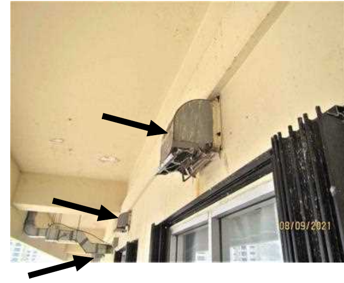
DETERIORATED WALL EXHAUST HOOD (3ea.).
