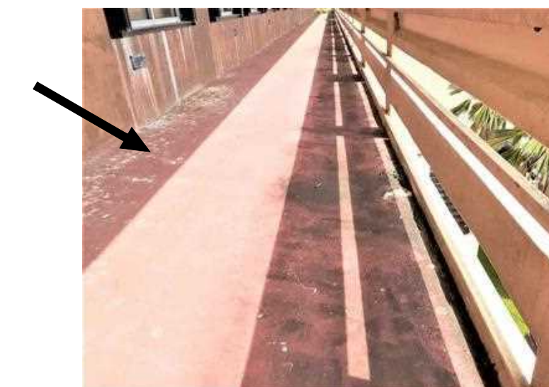
DETERIORATED FLOOR COATING MEMBRANE (640 sf).
