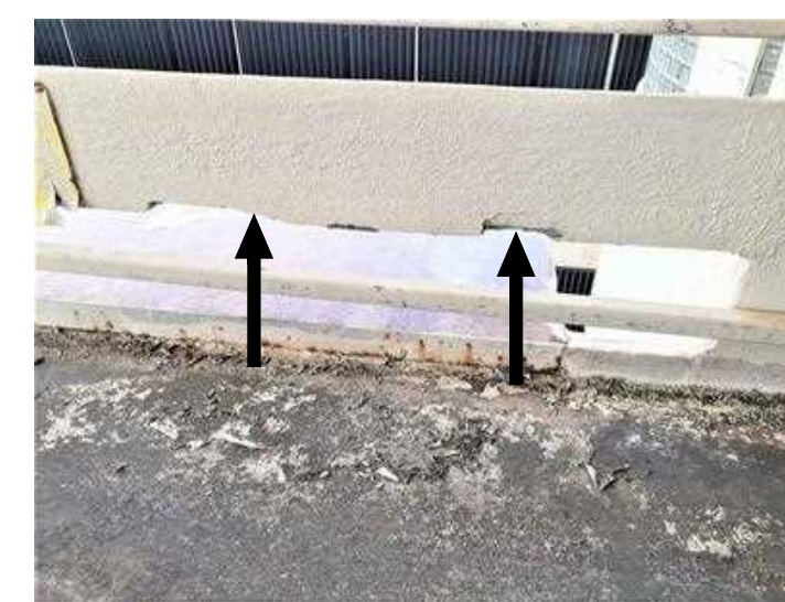
CONC RAILING SPALLS (8 Lf x 6")
