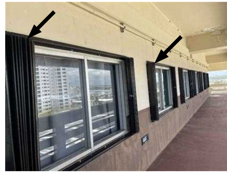
DETERIORATED WINDOW ACCORDION SHUTTERS (TYP 30 PLACES).
