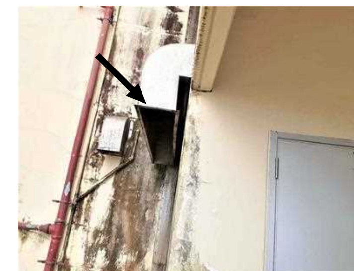
EXHAUST HOOD COVER MISSING
