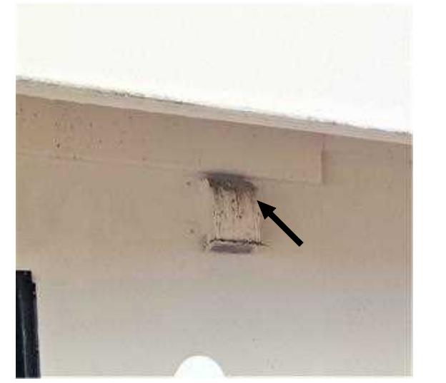
WALL MOUNTED EXHAUST HOOD RUSTED WITH BIRD DROPPING.
