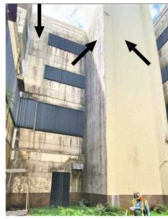
DETERIORATED EXISTING WALL PAINTS (900 sf).
