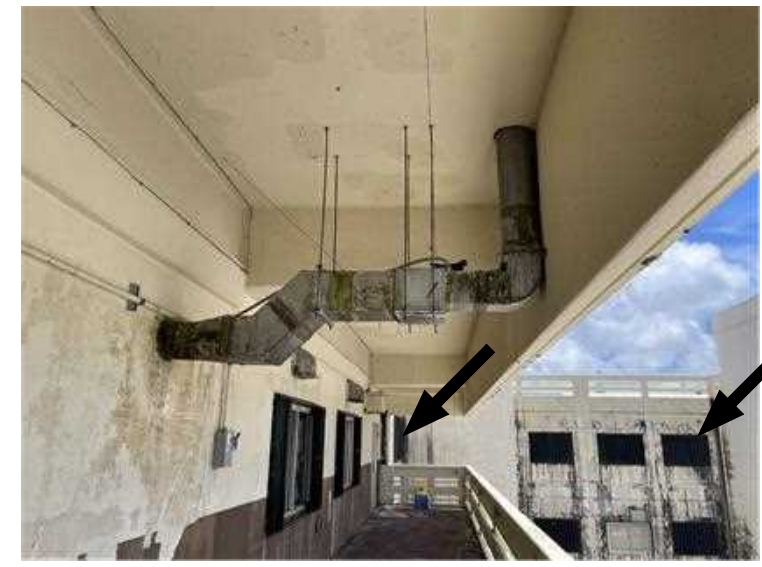
DETERIORATED WINDOW SHUTTERS (TYP 10 PLACES).
