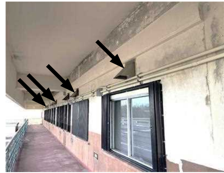
DETERIORATED WALL EXHAUST HOOD.
