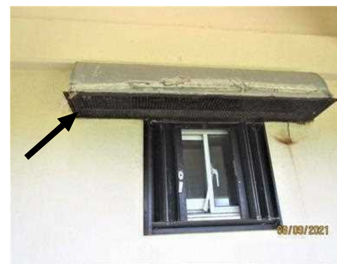
DETERIORATED WALL EXHAUST HOOD
