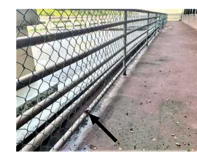
DETERIORATED CHAIN LINK & PIPE RAILING & ITS ACCESSORIES (158 lf).
