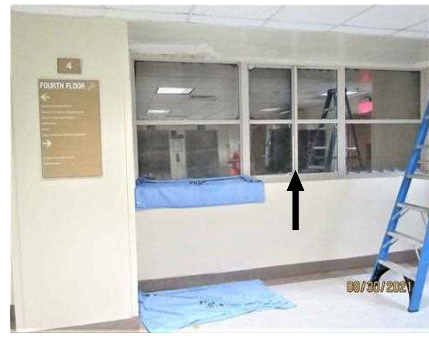
DETERIORATED GLASS WINDOW AND FRAMES
