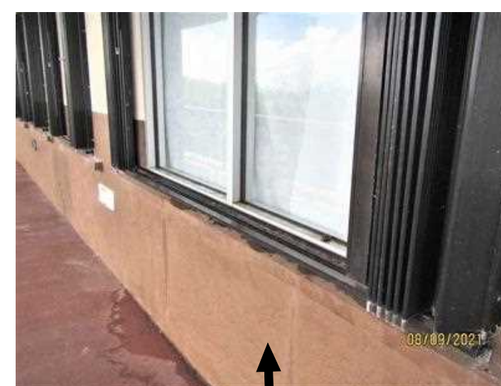
DETERIORATED WALL PAINT (3,510 Sf)
