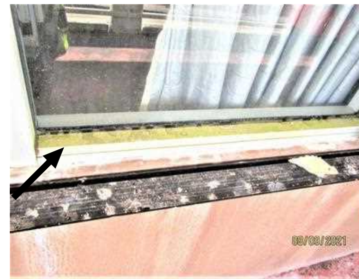
MILDEW WITH MOISTURE ON WINDOW SILL (4-6'x4') (2-48"x32")
