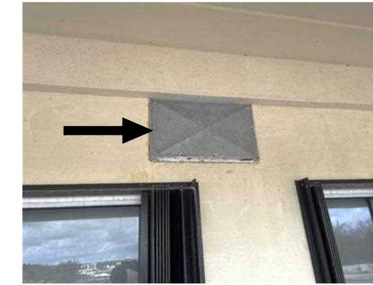
DETERIORATED EXHAUST/OUTSIDE AIR GRILLE COVER.
