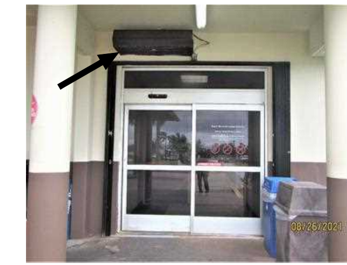
DETERIORATED DOOR HEAD BLOWER.
