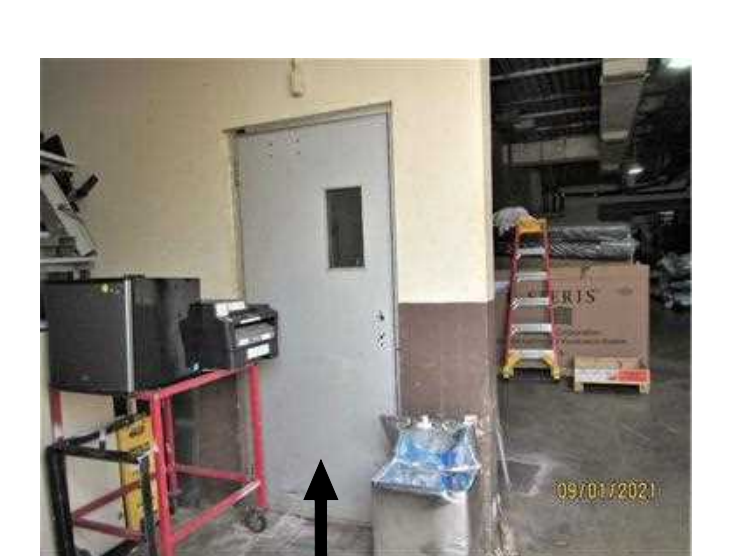
DETERIORATED SINGLE DOOR INCLUDING ACCESSORIES.
