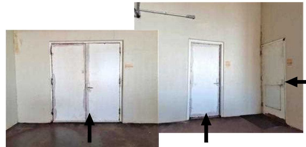
DETERIORATED DOORS, SEALANT (108 Lf), SEAL (62Lf) & DOOR THRESHOLD (12 Lf).
