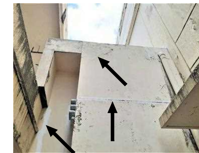
WALL HAIRLINE CRACKS (8 Lf).
