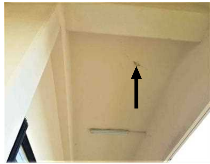
CEILING CRACKS (5 lf).
