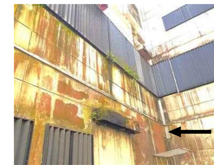
DETERIORATED SEISMIC JOINT COVER (FLOOR, SIDES & CEILING) (36 lf).
