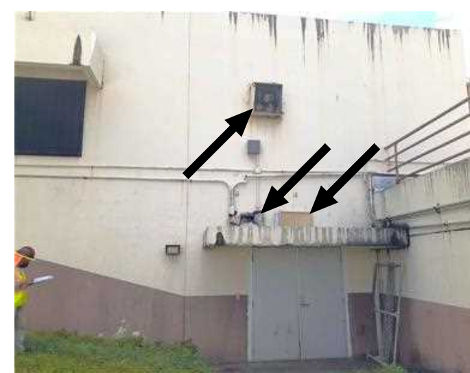
DETERIORATED WALL EXHAUST and WALL OPENING COVER MISSING.
