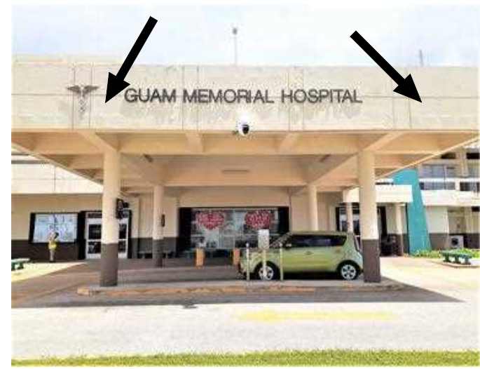
DETERIORATED WALL PAINT AT PARAPET (544 sf).
