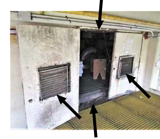
MECHANICAL EQUIPMENT DOOR BROKEN & RUSTED (2 ea).
