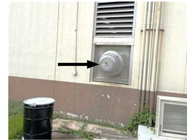
DETERIORATED WALL EXHAUST HOOD.
