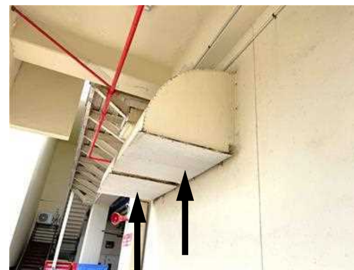
DETERIORATED EXHAUST HOOD
