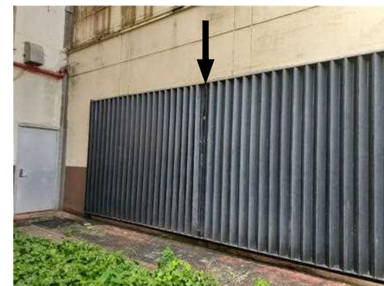
DETERIORATED WINDOW SHUTTERS
