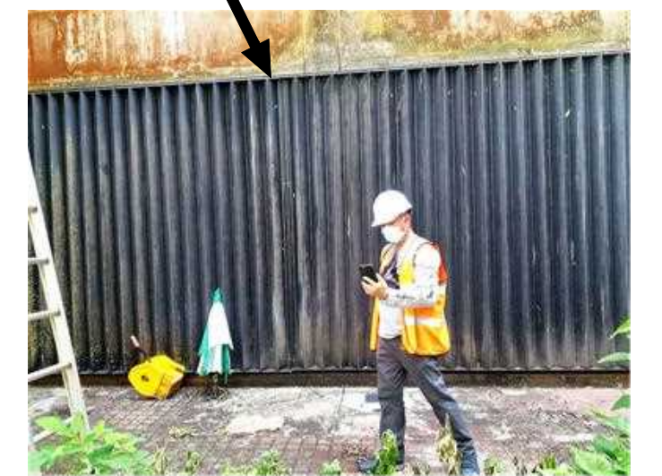
DETERIORATED WINDOW SHUTTERS
