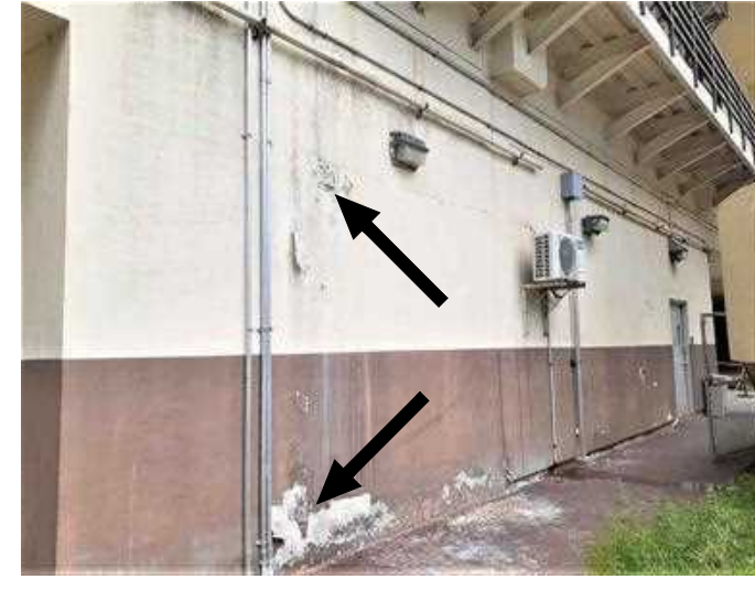
CONCRETE DAMAGED ON WALL (14 Sf).
