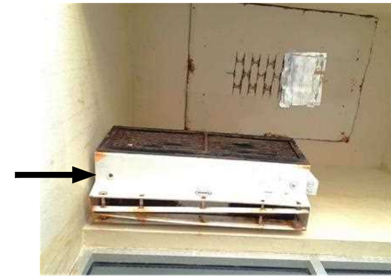
DETERIORATED DOOR HEAD BLOWER.
