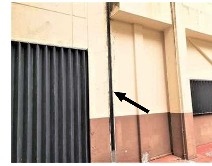
CORRODED METAL CHANNEL AND WALL SEISMIC JOINT (38 lf).
