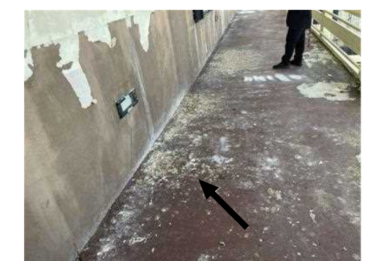
BIRDS DROPPINGS PRESENT ON BEAM, HOODS, PIPES, DUCT WORK, SHUTTER HEAD, ETC. FROM LIGHT TO HEAVILY INFESTED NARROW TO EXTRA WIDE AREAS.
