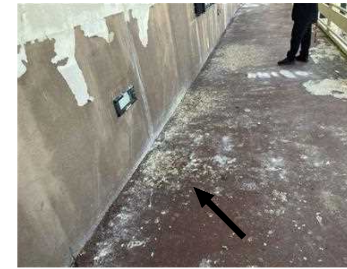
BIRDS DROPPINGS PRESENT ON BEAM, HOODS, PIPES, DUCT WORK, SHUTTER HEAD, ETC. FROM LIGHT TO HEAVILY INFESTED NARROW TO EXTRA WIDE AREAS.
