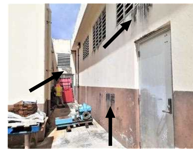
DETERIORATED WALL PAINTS (900 sf).
