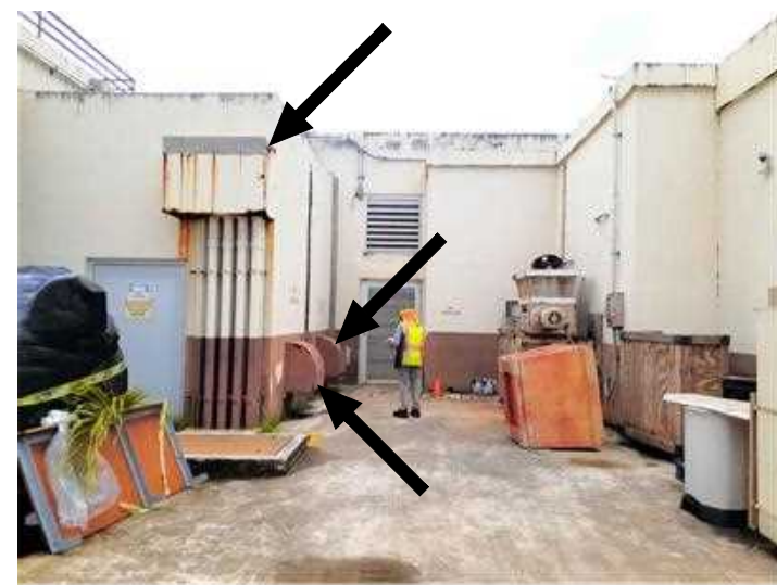
DETERIORATED METAL HOODS (3 ea).
