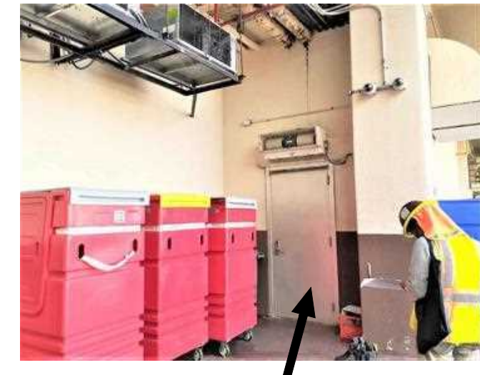
FAILED DOOR Seal, THRESHOLD AND SealANT (20 lf).
