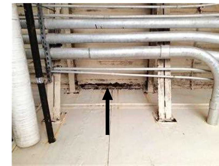
DETERIORATED and RUSTED METAL DECKING (597 sf).
