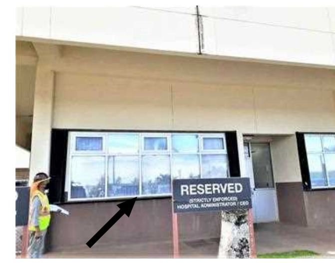
DETERIORATED WINDOW SeaLANT AND Seal (644 lf).
