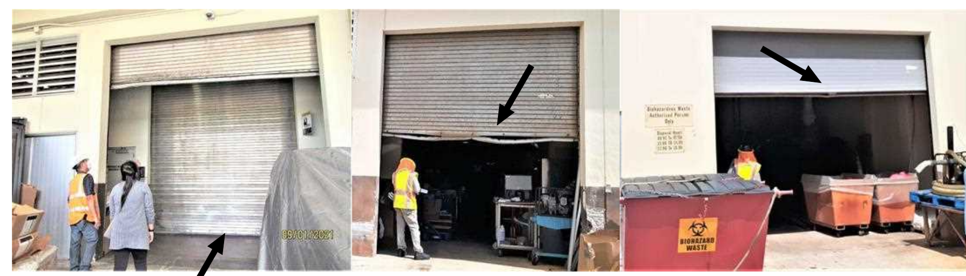
DETERIORATED OR DAMAGED ROLL-UP DOORS, 5 ea (654 sf).
