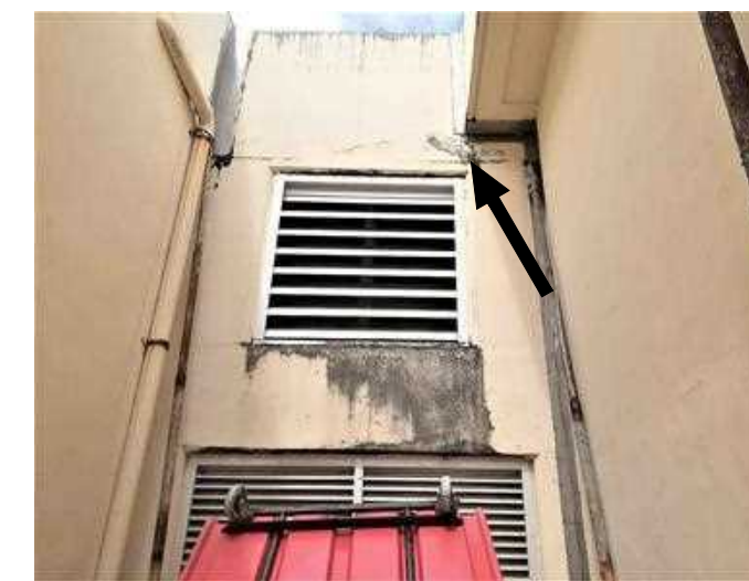
CONCRETE WALL SPALLS AND CRACKS
