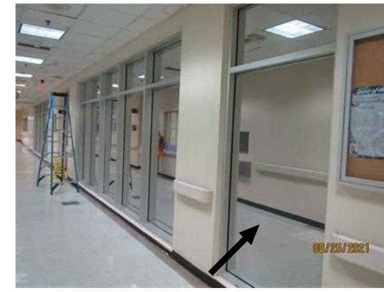
DETERIORATED FIXED GLASS WINDOW CURTAIN WALL.
