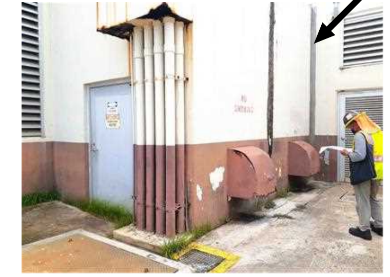
DETERIORATED CONSTRUCTION JOINT COVER (10 lf).
