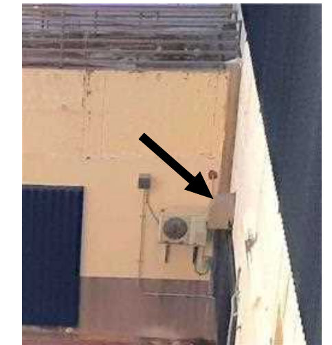
DETERIORATED EXHAUST HOOD
