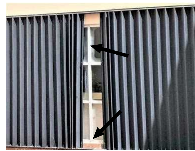
DETERIORATED WINDOW SEALANT (112 lf) and SEAL (368 lf).
