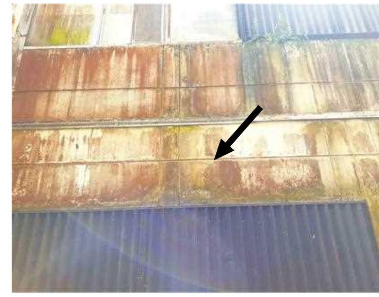
DETERIORATED WALL PAINT w/ CRACKS (476 sf).
