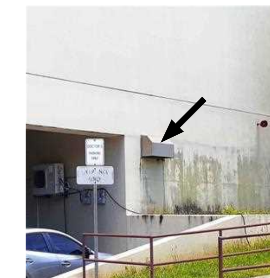
DETERIORATED WALL EXHAUST HOOD.
