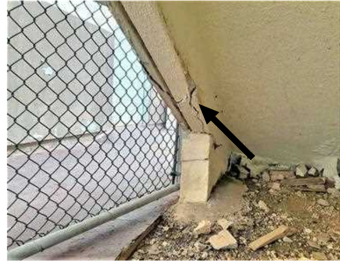
BELOW STAIR CRACKS AND SPALLS (5 Lf & 3 Sf).
