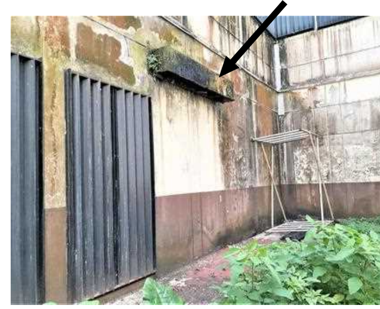
DETERIORATED WALL EXHAUST HOOD w/ VEGETATION (1 ea).
