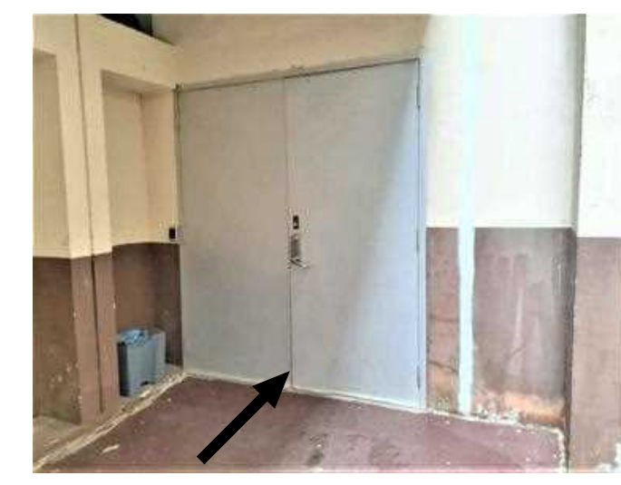
DETERIORATED DOOR WITH WATER LEAK
