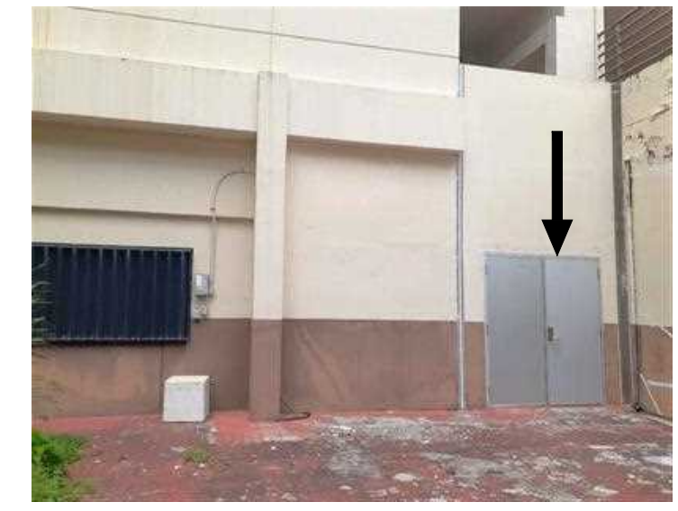
DETERIORATED DOOR, SEAL, SEALANT and THRESHOLD.
