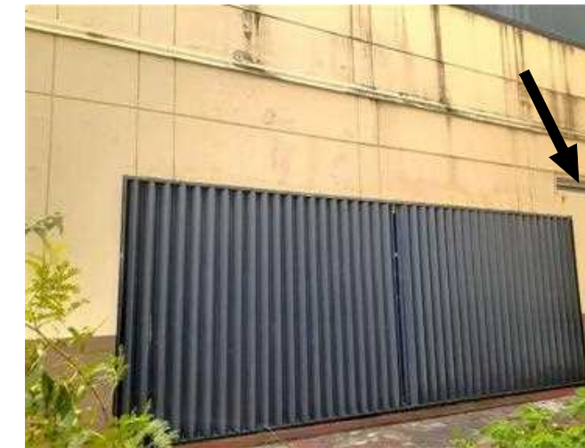
DETERIORATED MECHANICAL AIR INTAKE GRILLE on WALL
