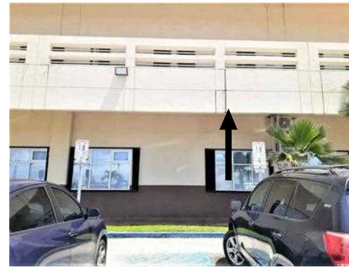
MOLD AND MILDEW ON FASCIA (1024 sf).
