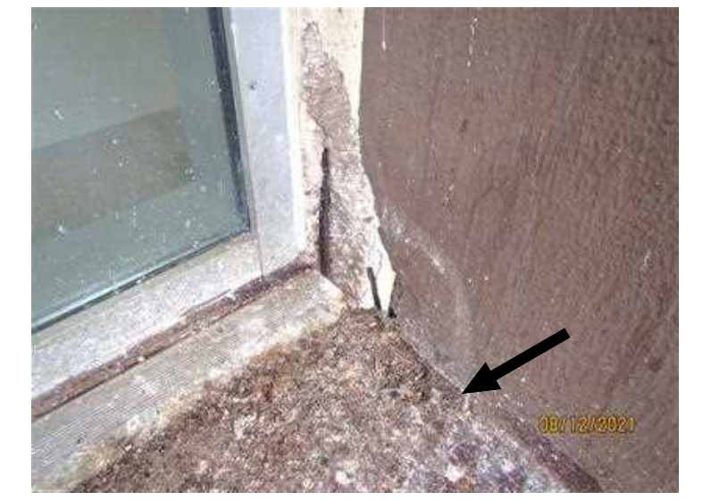
BIRDS DROPPINGS PRESENT ON BEAM, HOODS, PIPES, DUCT WORK, SHUTTER HEAD, ETC. FROM LIGHT TO HEAVILY INFESTED NARROW TO EXTRA WIDE AREAS.
