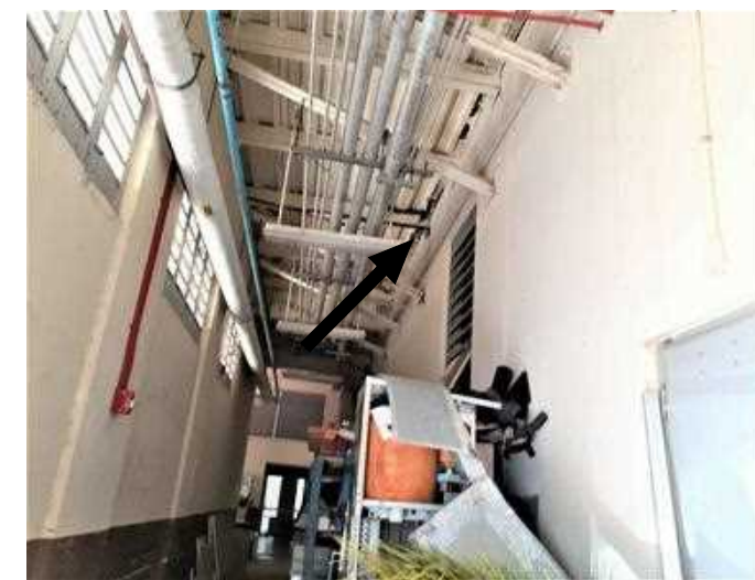
DETERIORATED AND RUSTED METAL DECKING (597 sf).
