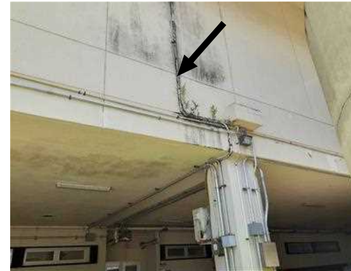
ELECTRICAL PIPE DETERIORATED.
