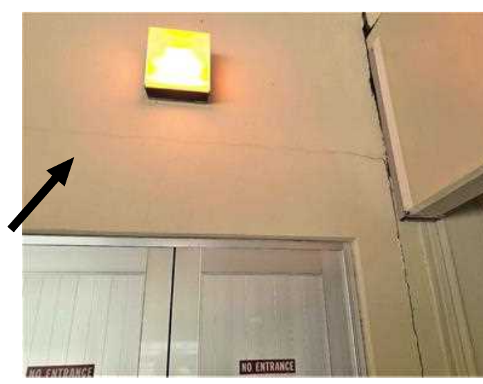
MOISTURE PRESENT ON CEILING & DETERIORATED PAINT (525 sf).
