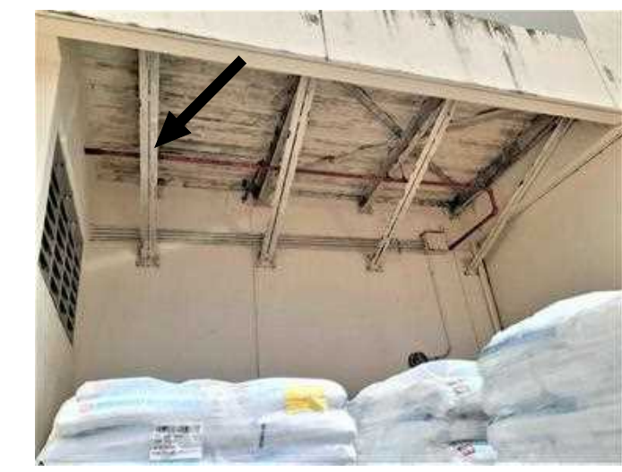
DETERIORATED STEEL ROOF TRUSSES (12 ea).
