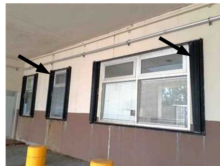
DETERIORATED WINDOW ACCORDION SHUTTERS
