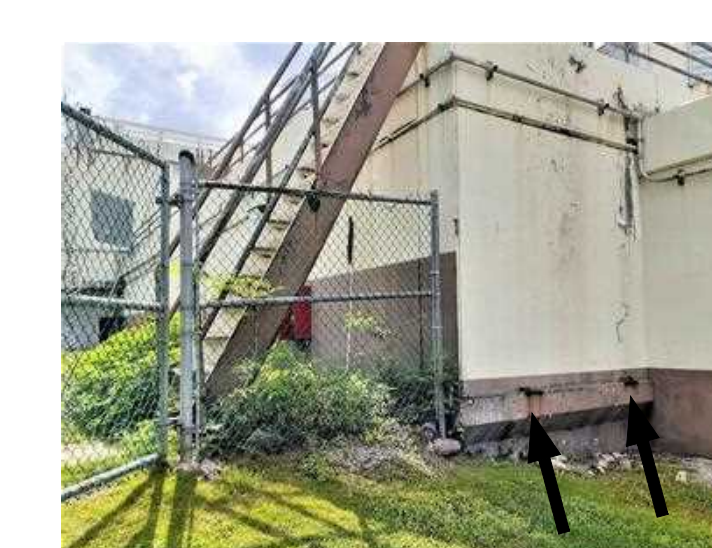
FLOOR GRADE BEAM SPALLS (2 sf).
