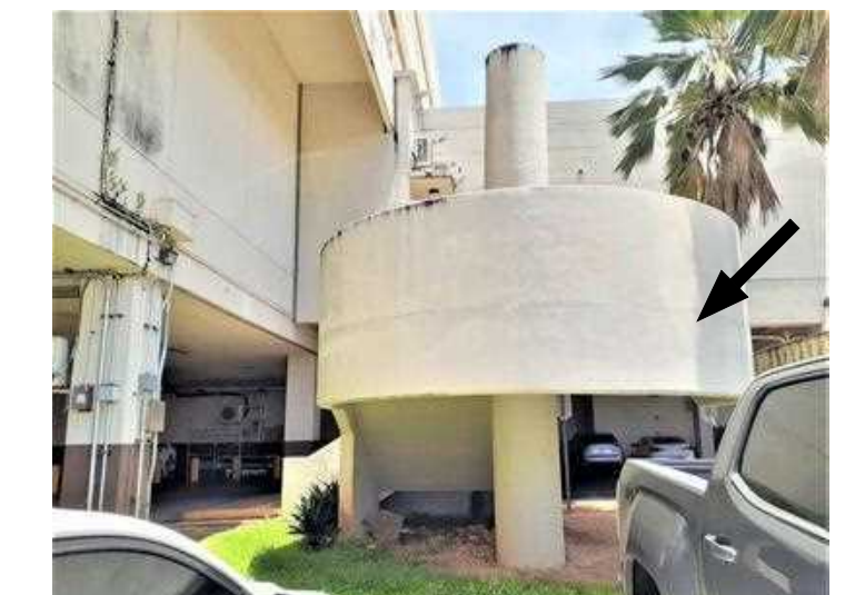
STAIR WALL CRACKS (30 Lf).
