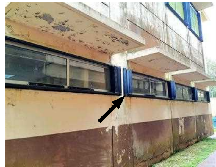
DETERIORATED WINDOW ACCORDION SHUTTERS
