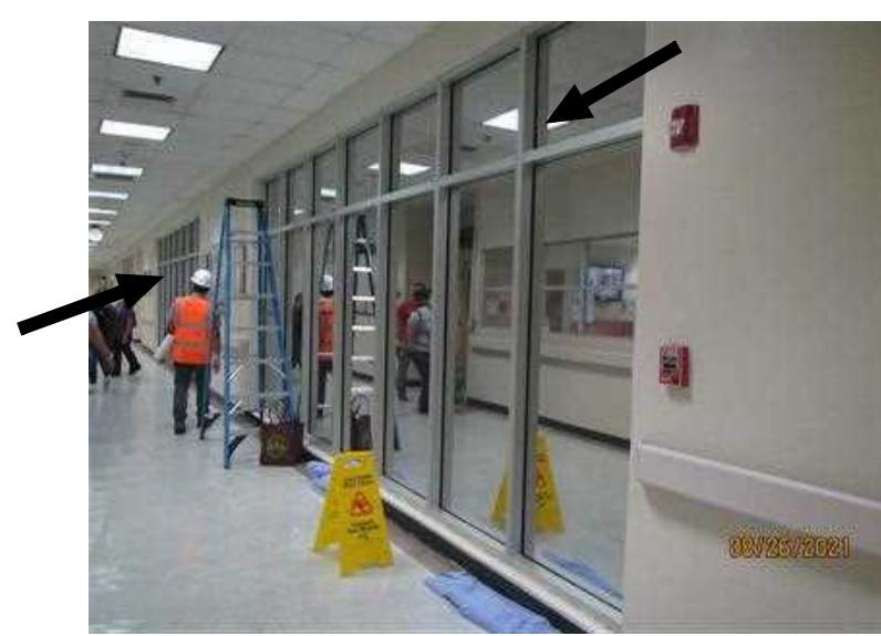
DETERIORATED GLASS CURTAIN WALLS, TYPICAL.
