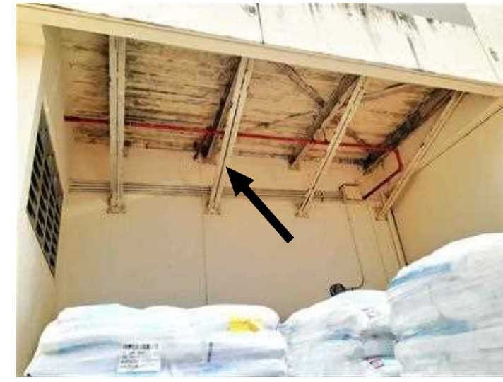
DETERIORATED STEEL ROOF TRUSSES (12 ea).
