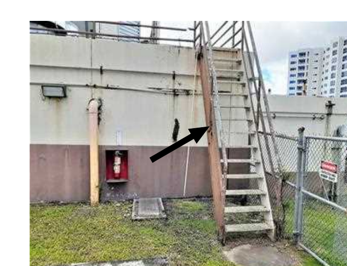
DETERIORATED ACCESS STEEL STAIRS.
