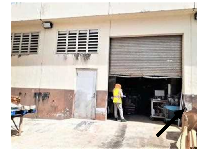
CONCRETE WALL SPALLS (16 sf).
