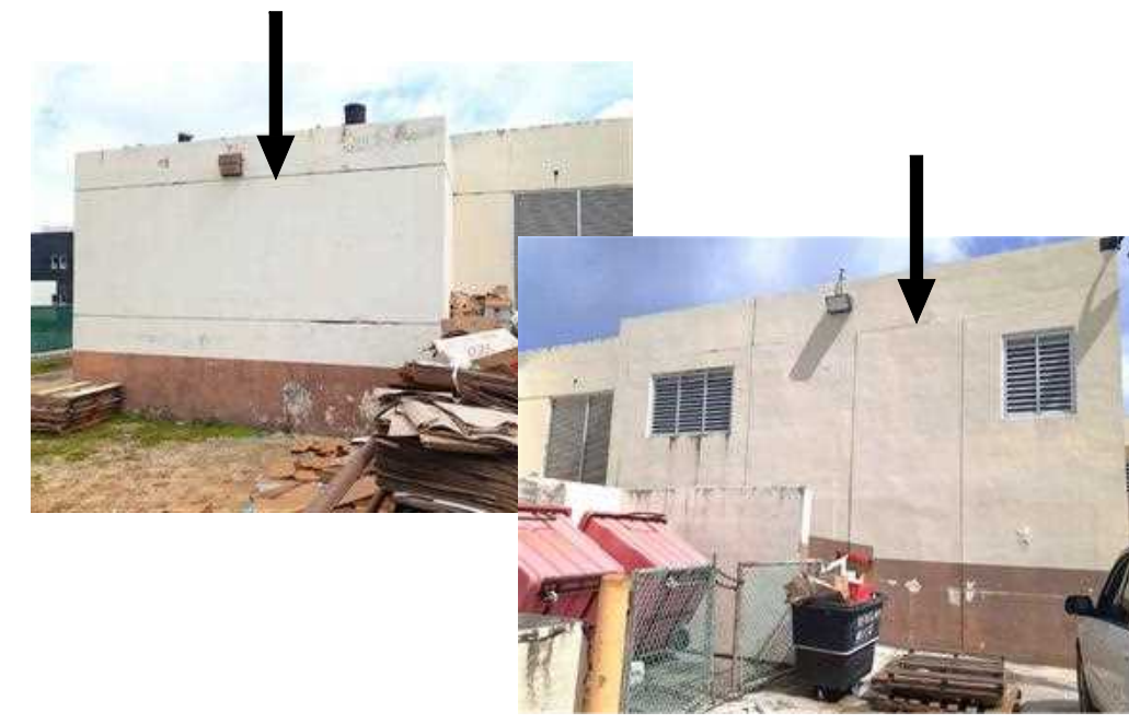
DETERIORATED WALL PAINTS (90 sf).
