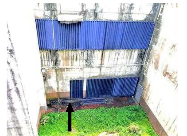
BIRDS DROPPINGS PRESENT ON BEAM, HOODS, PIPES, DUCT WORK, SHUTTER HEAD, ETC. FROM LIGHT TO HEAVILY INFESTED NARROW TO EXTRA WIDE AREAS.
