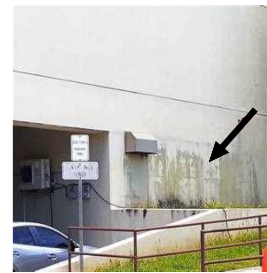
DETERIORATED WALL PAINT with MILDEW and ALGAE.
