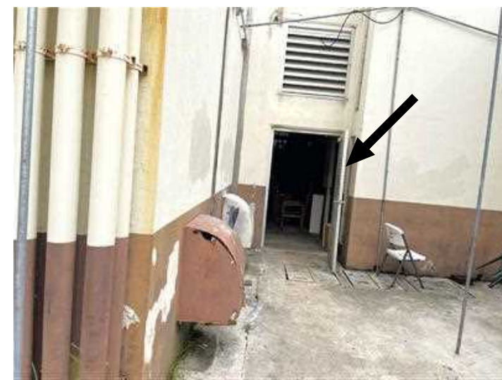
DETERIORATED LOUVERED DOOR
