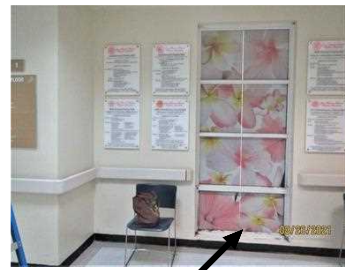
DETERIORATED GYPSUM BOARD AROUND WINDOW (24 sf).
