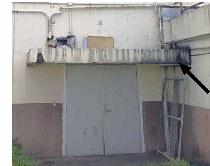
DETERIORATED CANOPY PAINTS.
