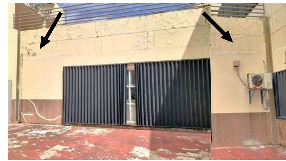
DETERIORATED WALL PAINT (663 sf).
