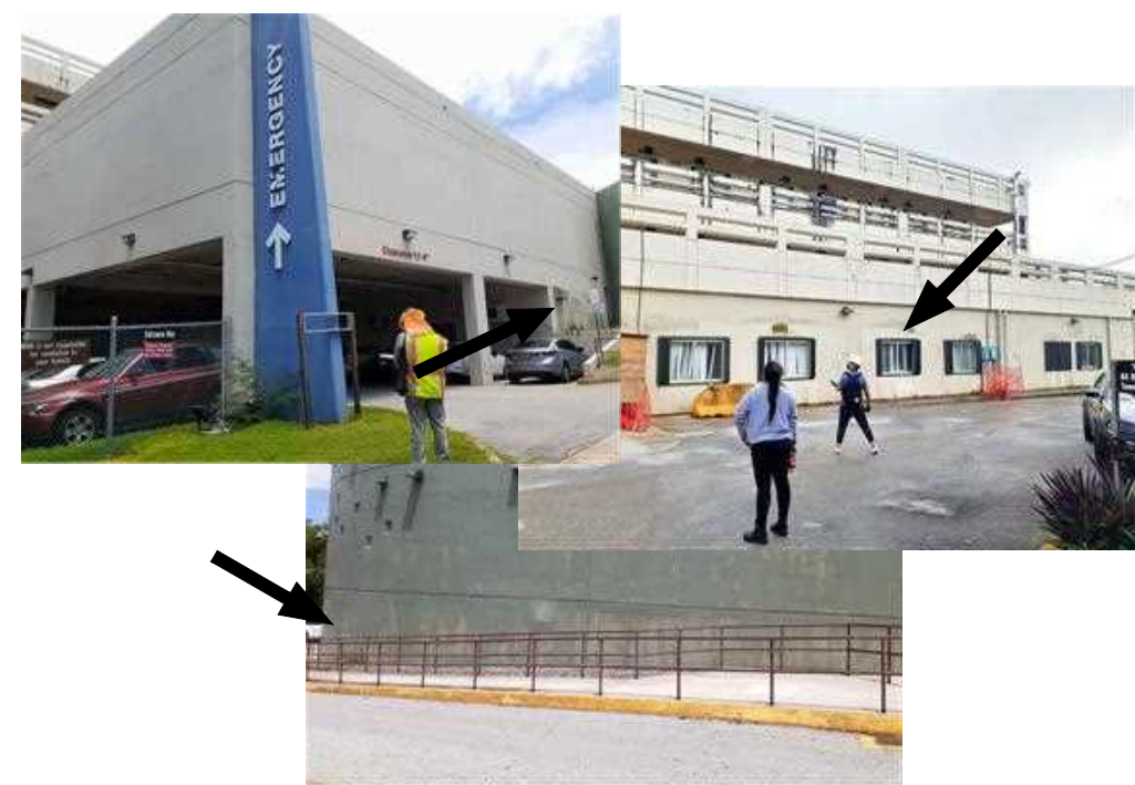
DETERIORATED WALL, and PARAPET WALL PAINTS.
