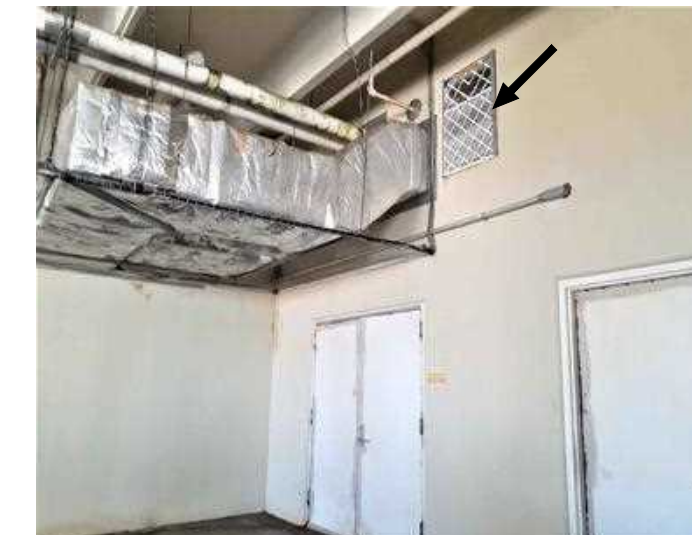
WALL OPENING DAMAGED COVER.
