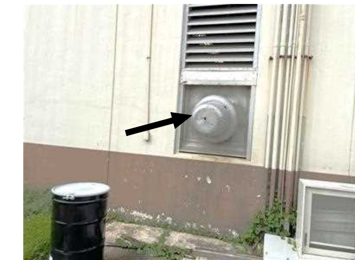
DETERIORATED EXHAUST HOODS.
