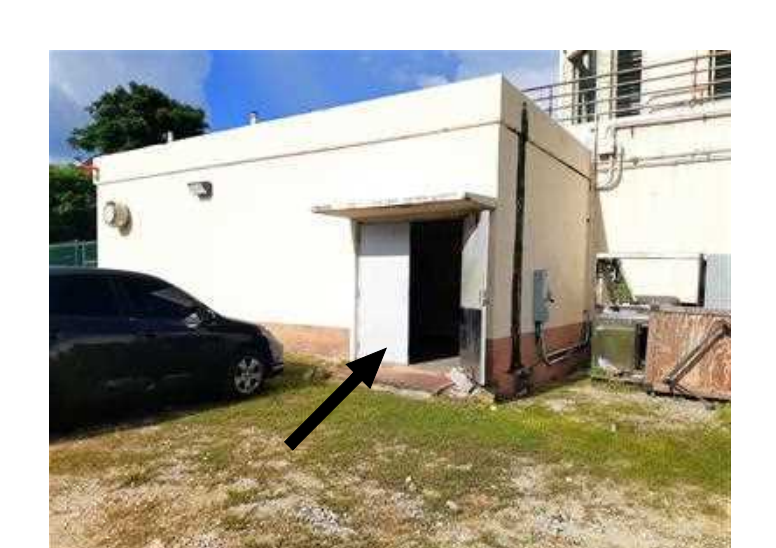
FAILED DAMAGED DOOR.
