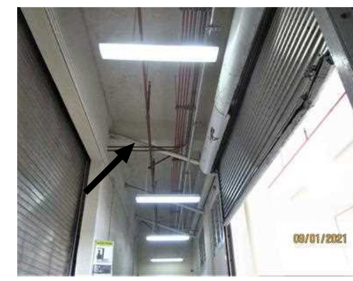
DETERIORATED STEEL TUBING WALL BRACE (6 ea).
