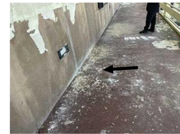
BIRDS DROPPINGS PRESENT ON BEAM, HOODS, PIPES, DUCT WORK, SHUTTER HEAD, ETC. FROM LIGHT TO HEAVILY INFESTED NARROW TO EXTRA WIDE AREAS.
