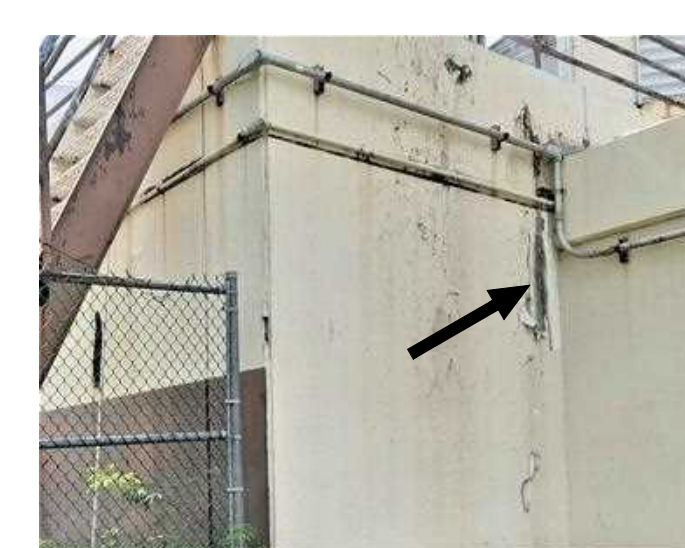
WALL PAINT FLAKING (52 sf).
