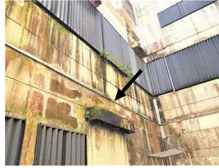
DETERIORATED METAL FLASHING (30 lf).
