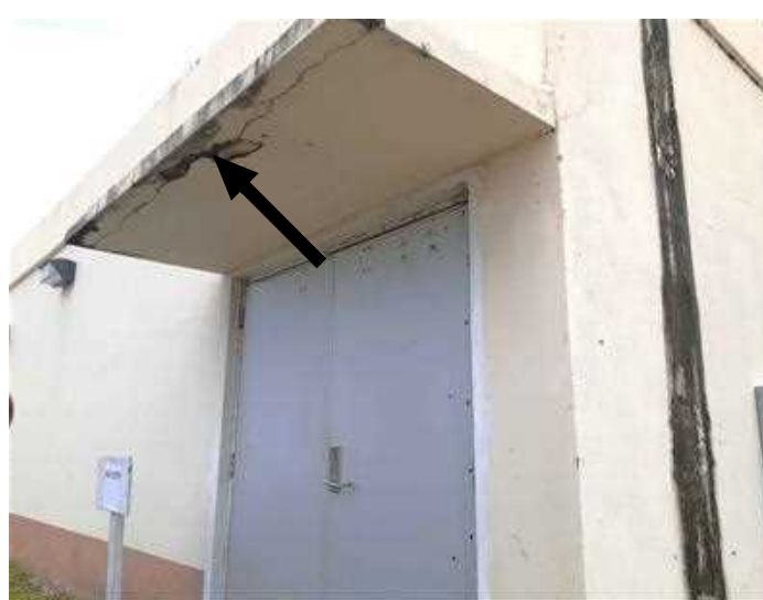
CONCRETE CRACKS & SPALLS ON CANOPY.
