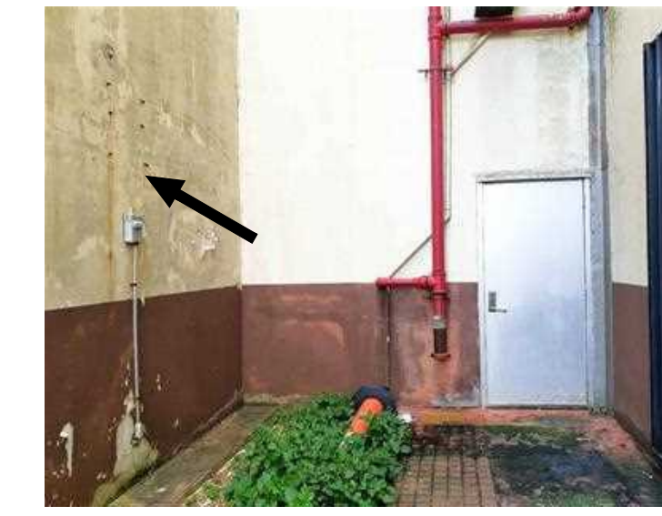
DETERIORATED WALL PAINT w/ MULTIPLE CRACKS (Cracks 30 lf), (WALL 260 sf)
