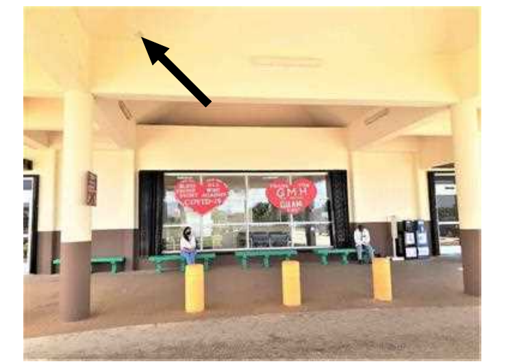
DETERIORATED CEILING PAINT (12 sf).
