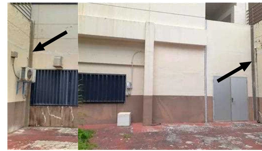
DETERIORATED SEISMIC JOINT COVER (FLOOR, SIDES & CEILING) (36 lf).
