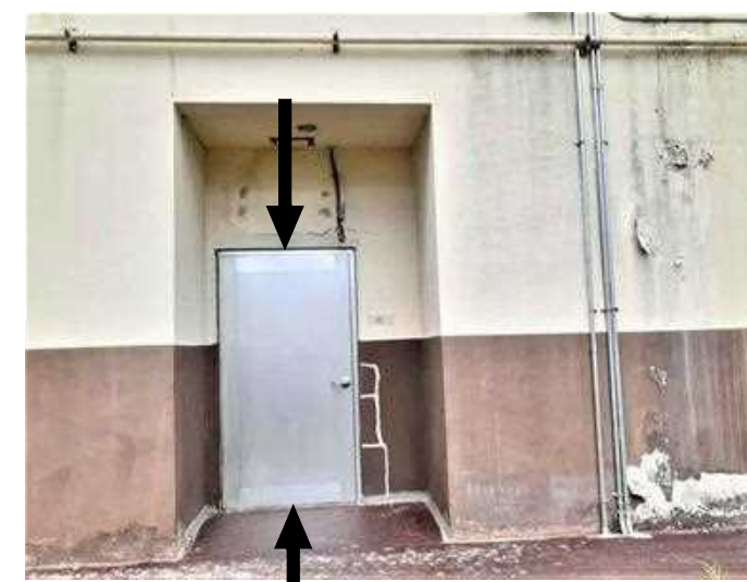
DETERIORATED DOOR THRESHOLD (6 lf).
