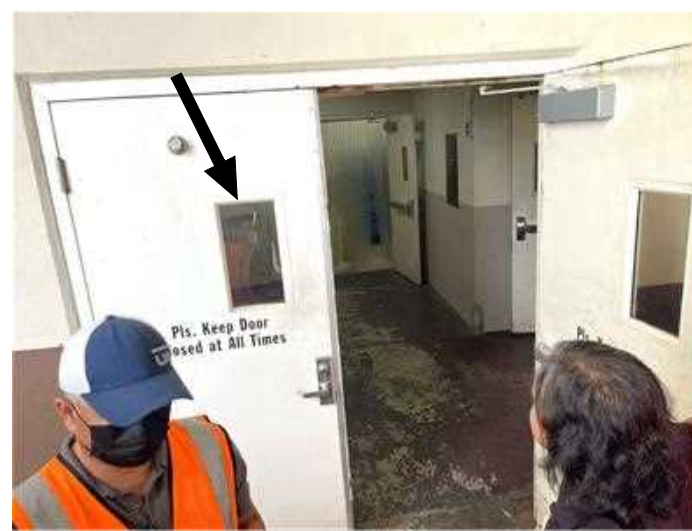
DETERIORATED DOOR with VISION PANEL
