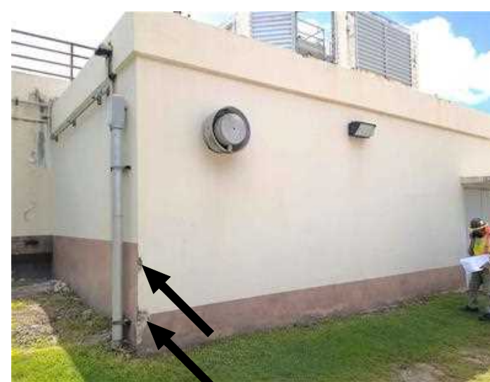
CORNER SPALLS (2 lf).
