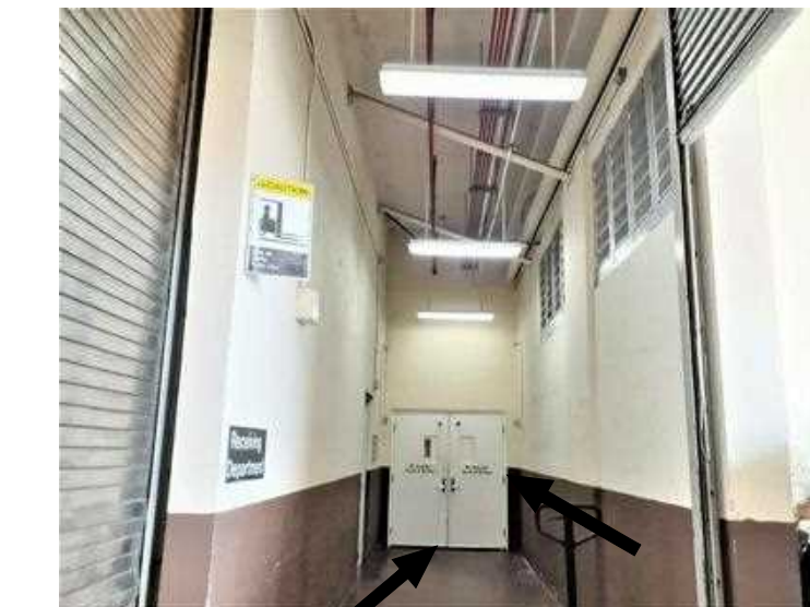
DETERIORATED DOOR THRESHOLD (6 lf). FAILED DOOR SEAL (40 lf).
