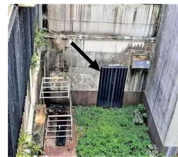
DETERIORATED WINDOW SHUTTERS
