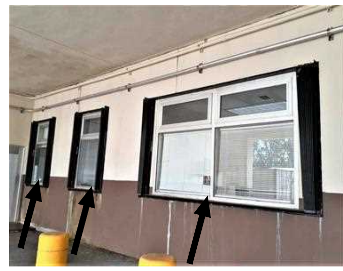
DETERIORATED WINDOW SEALANT AND SEAL
