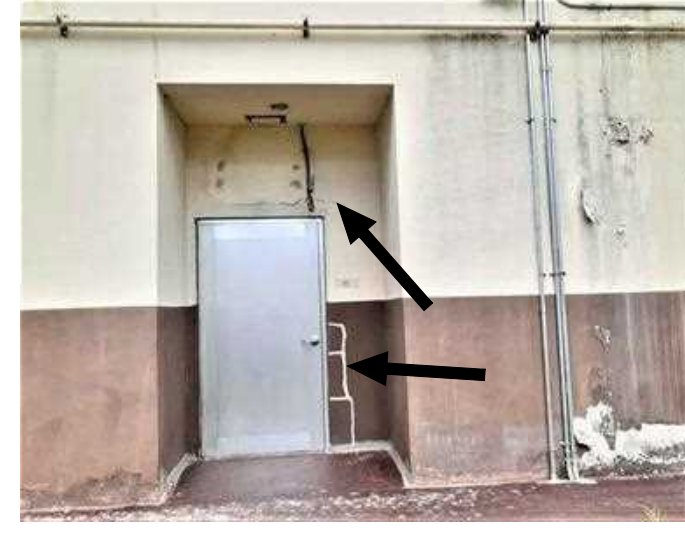
CONCRETE WALL CRACKS (12 Lf).
