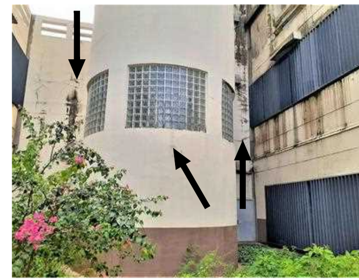
DETERIORATED WALL PAINTS w/ CRACKS (1,326 sf).
