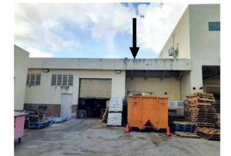
DETERIORATED PERIMETER PARAPET PAINT
