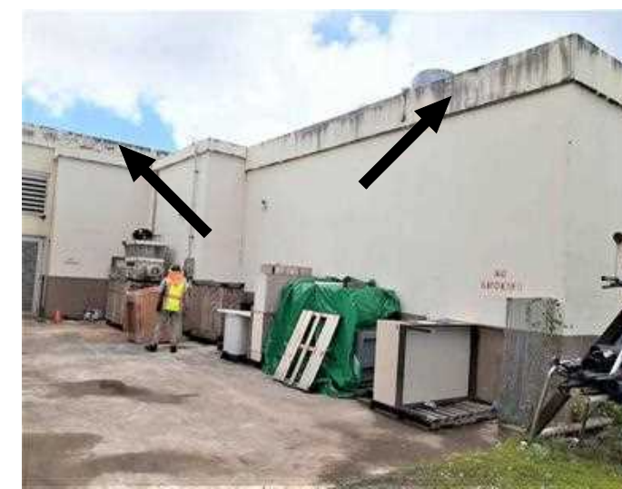
DETERIORATED PERIMETER PARAPET PAINT, TYPICAL.
