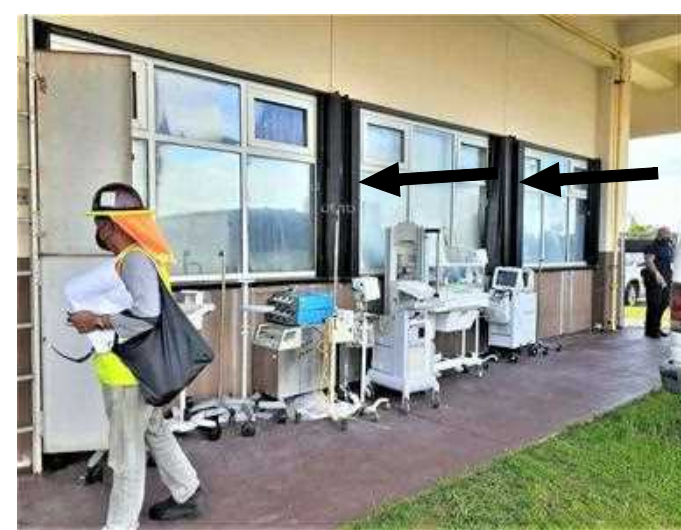
DETERIORATED WINDOW ACCORDION SHUTTERS
