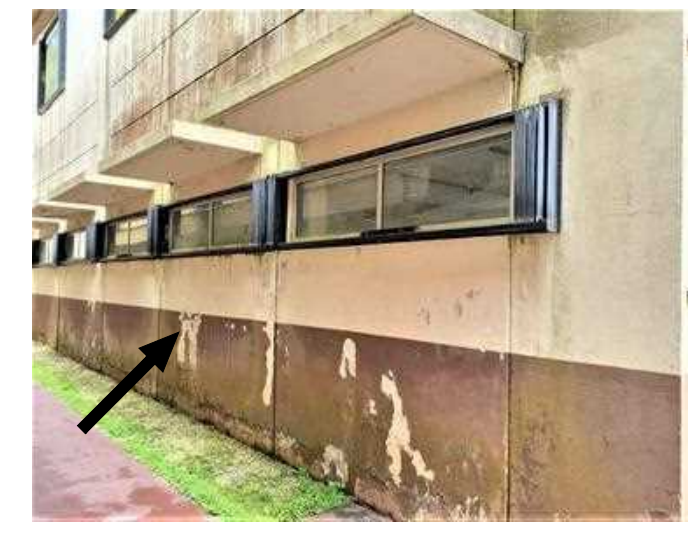
DETERIORATED WALL PAINT (780 Sf).
