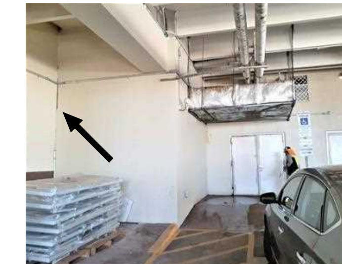
WALL CORNER SPALLS W/ EXPOSED REBAR (12 Lf), (6 Sf).
