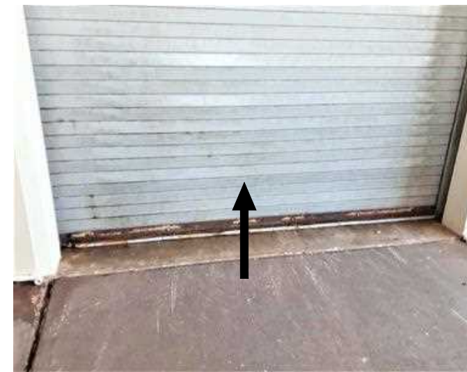
DETERIORATED ROLL-UP DOOR (128 Sf).
