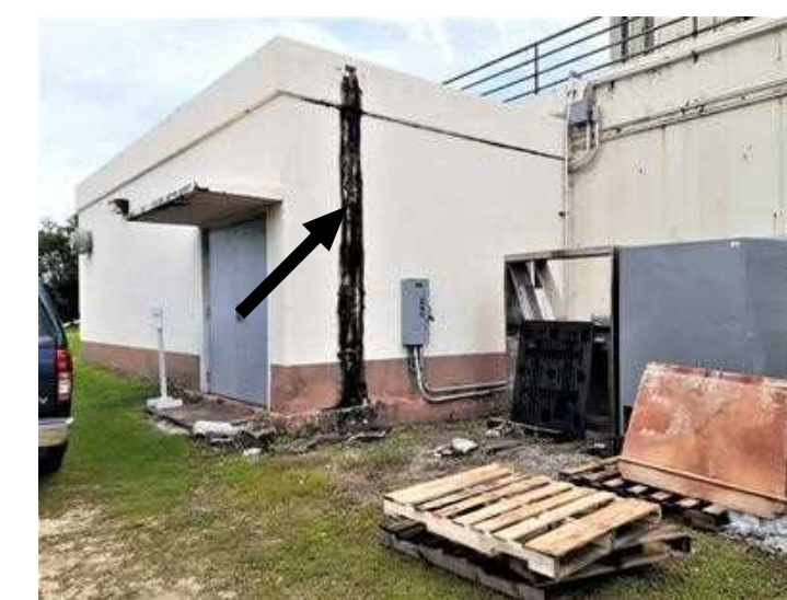
SEVERE MILDEW AT WALL (180 sf).
