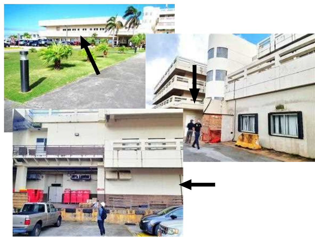
DETERIORATED WALLS, and PARAPET WALL PAINTS.
