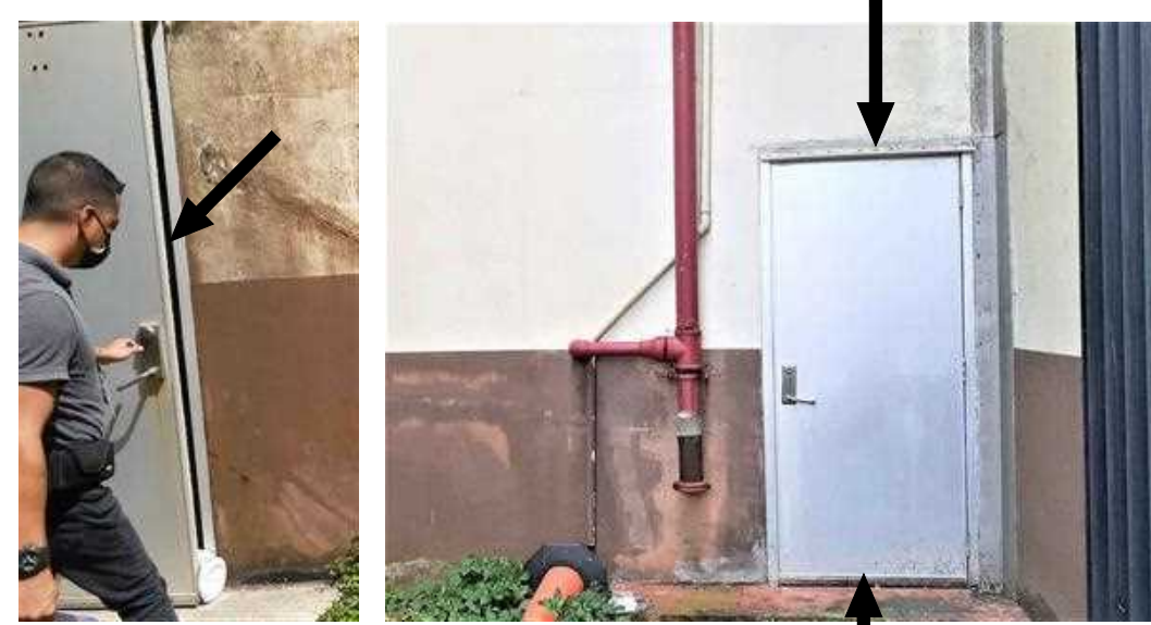
DETERIORATED DOOR, SEAL, SEALANT and THRESHOLD.
