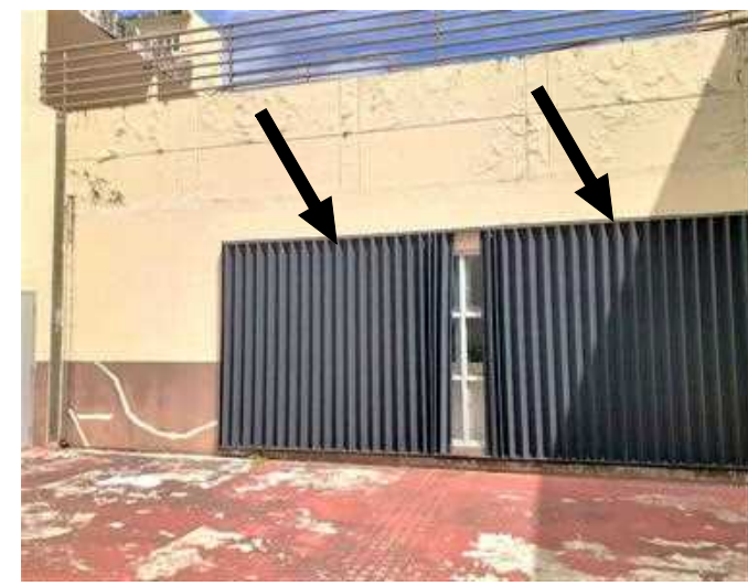
DETERIORATED EXISTING TYPHOON SHUTTERS.
