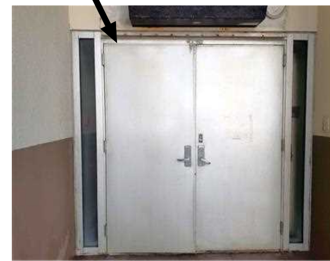
DETERIORATED DOOR with FIXED WINDOW SIDE PANEL
