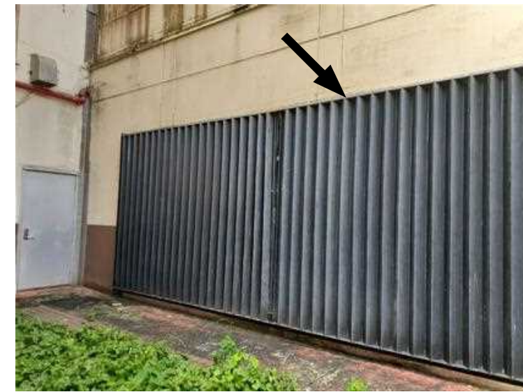
DETERIORATED WINDOW SHUTTERS
