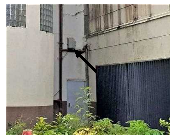
DETERIORATED WALL EXHAUST HOOD EQUIPMENT
