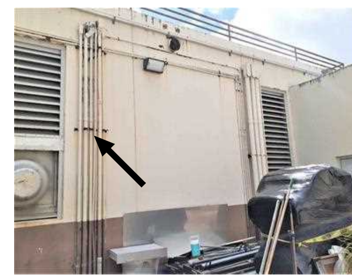
DETERIORATED ELECTRICAL CONDUITS with MILDEWS.
