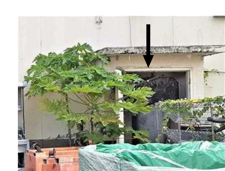
DAMAGED DOOR, HEADER & ACCESSORIES w/ CONCRETE SPALLS ON WALL & ROOF CANOPY.
