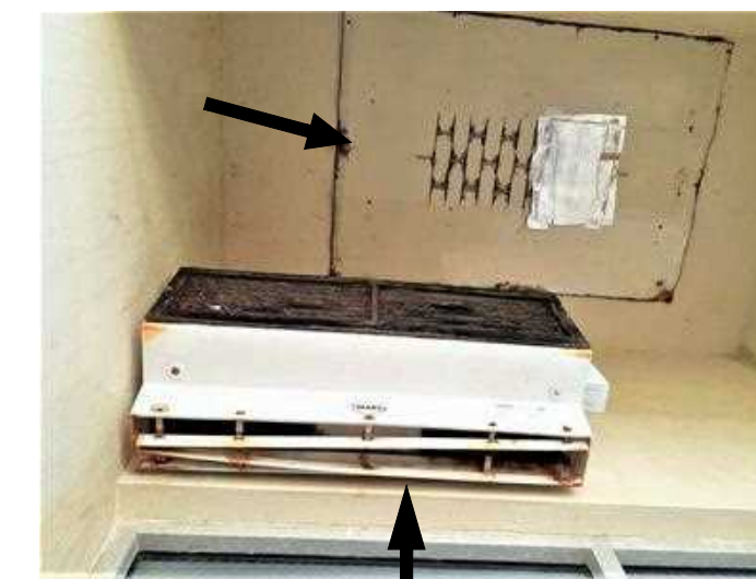
DETERIORATED DOOR HEAD BLOWER, and CEILING ACCESS DOOR HATCH.
