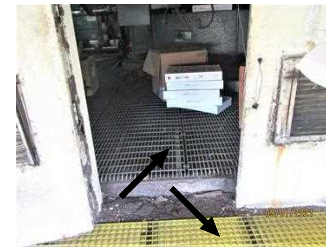
DETERIORATED MEZZANINE FLOOR GRATING (150 sf).
