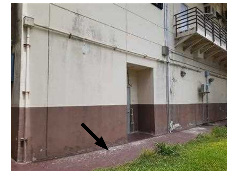
BIRDS DROPPINGS PRESENT ON BEAM, HOODS, PIPES, DUCT WORK, SHUTTER HEAD, ETC. FROM LIGHT TO HEAVILY INFESTED NARROW TO EXTRA WIDE AREAS.
