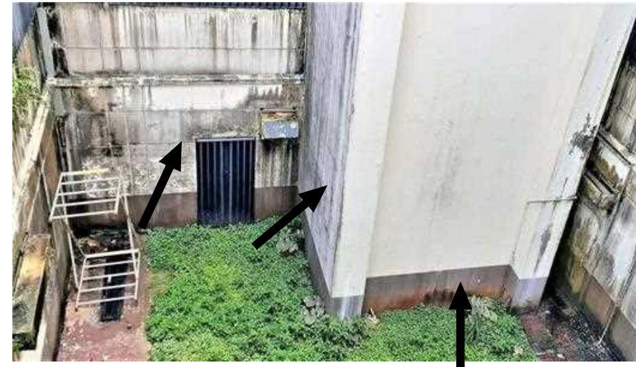
DETERIORATED WALL PAINTS (850 sf).
