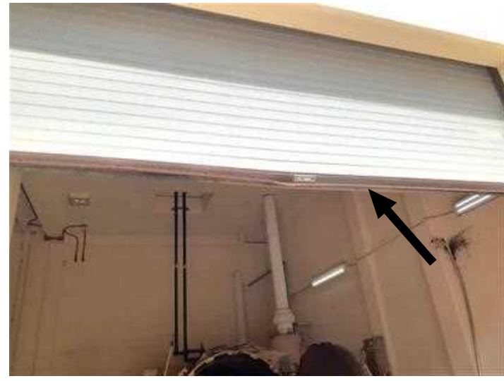
DETERIORATED OR DAMAGED ROLL-UP DOORS.
