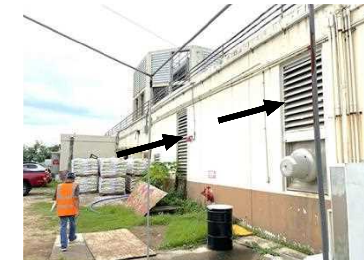
DETERIORATED WINDOW LOUVERS.
