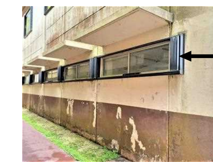
DETERIORATED ACCORDION WINDOW SHUTTERS
