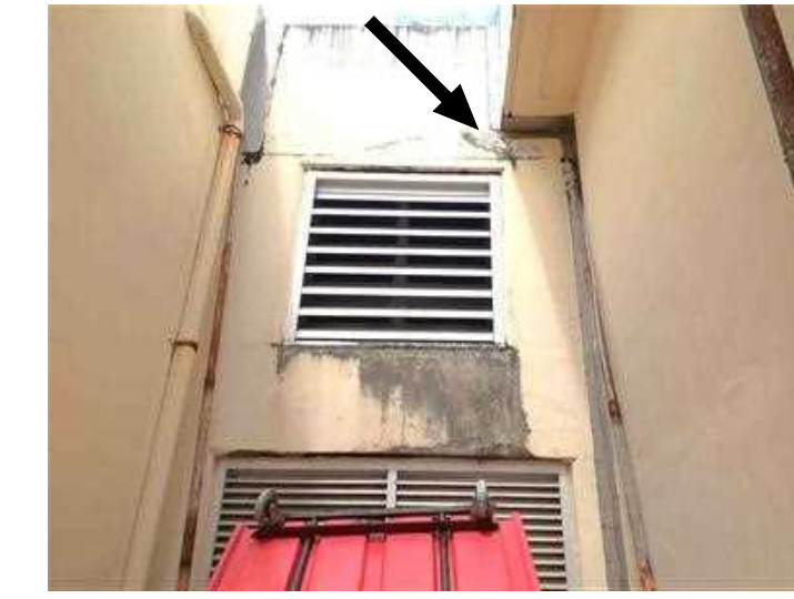
CONCRETE WALL SPALLS AND CRACKS (24 Sf).
