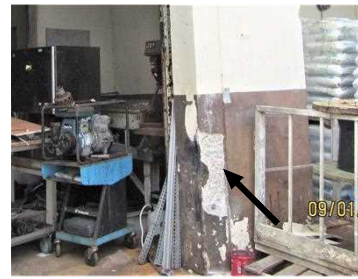
DETERIORATED WALL PAINT w/ CONCRETE CORNER SPALLS (16 sf).
