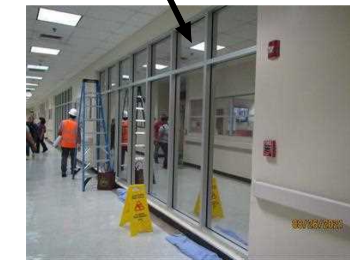
DETERIORATED DOOR with FIXED GLASS WINDOW CURTAIN WALL
