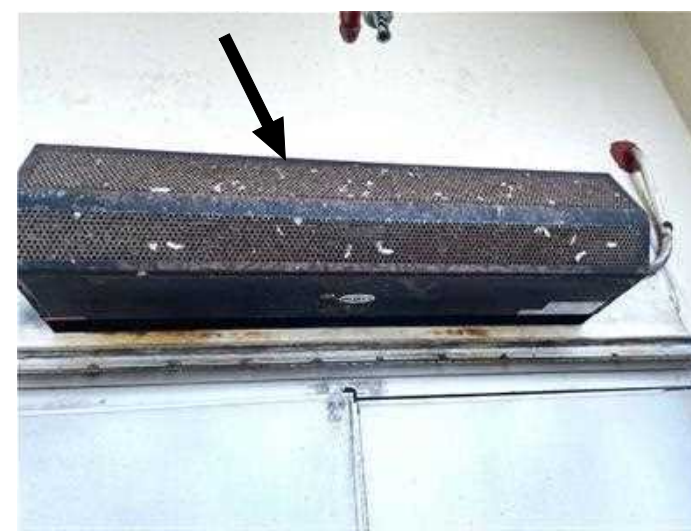
DETERIORATED DOOR HEAD BLOWER
