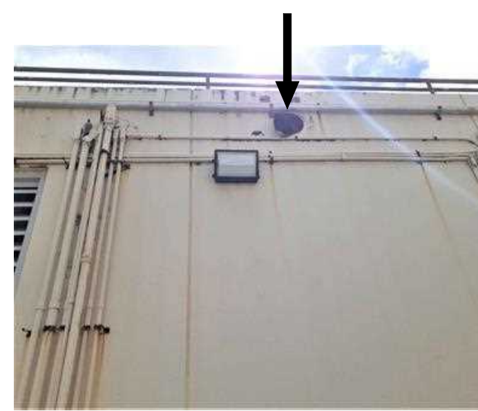
WALL EXHAUST MISSING
