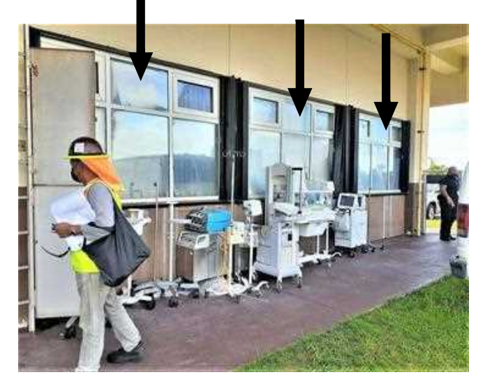
WINDOW STAINED AND MILDEW (324 sf).
