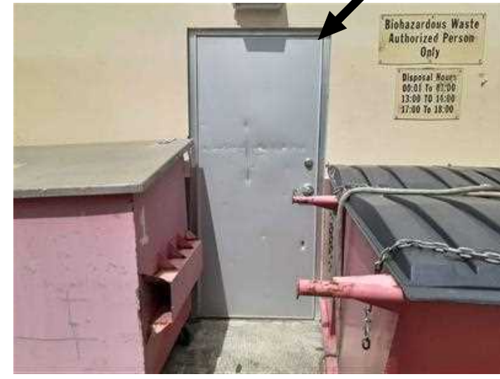
DETERIORATED SINGLE DOOR INCLUDING ACCESSORIES (3 ea).
