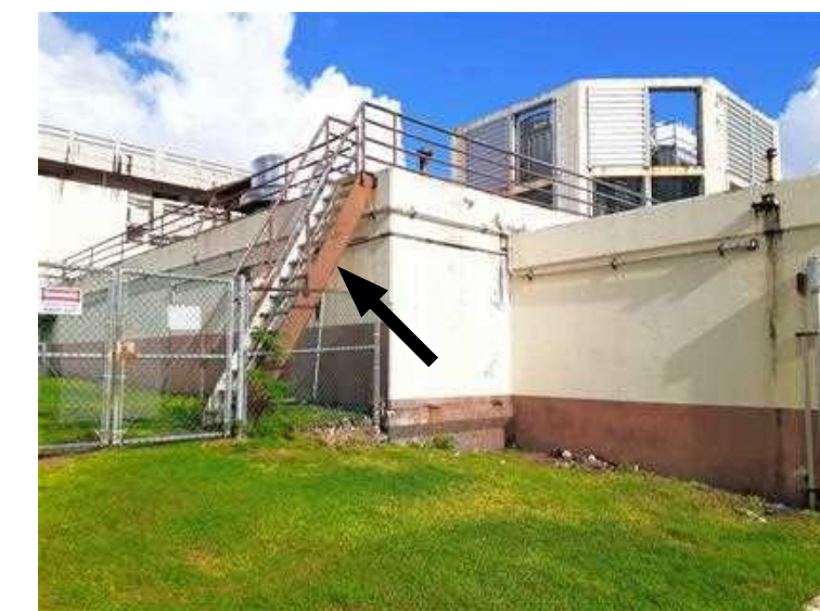
DETERIORATED ACCESS STEEL STAIRS.
