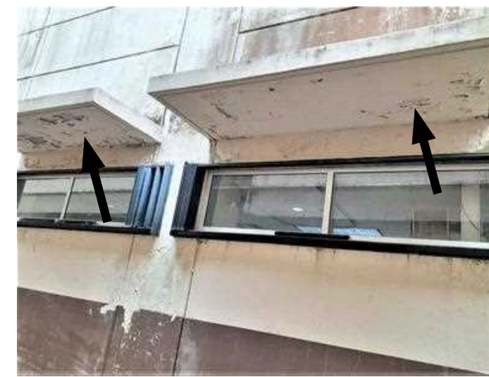
PAINT FLAKING ON CANOPY SOFFIT, TYP 6 PLACES (144 Sf).
