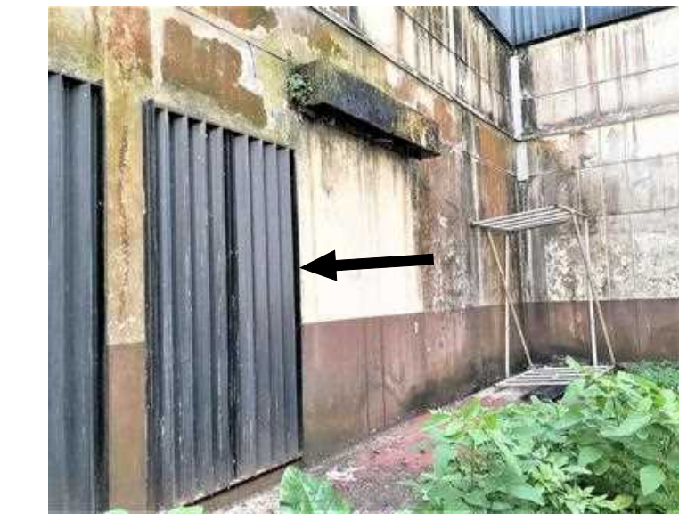
DETERIORATED WINDOW SHUTTERS
