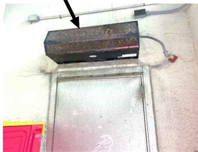
DETERIORATED DOOR HEAD BLOWER
