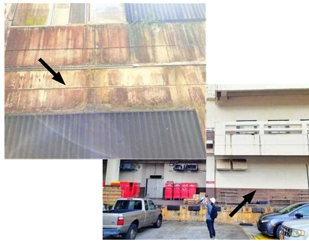
DETERIORATED WALL PAINTS (6,239 sf).
